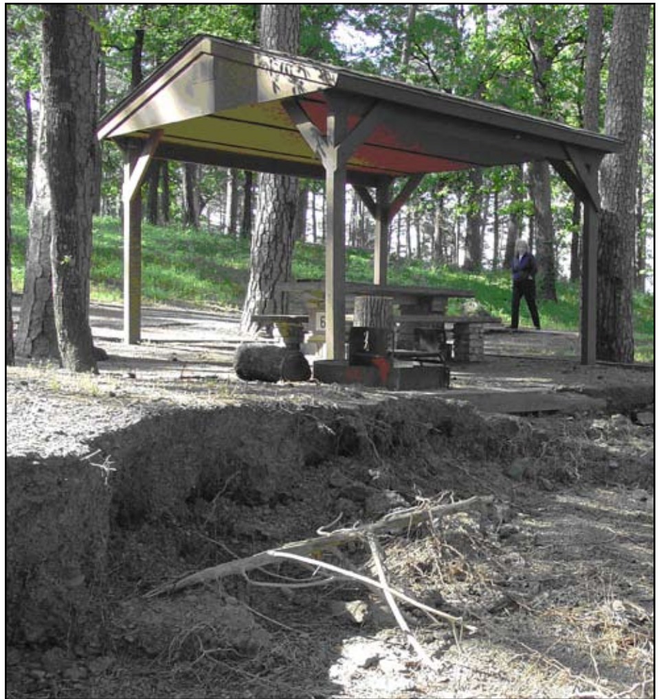
The erosion at this camp site in a Blue Mountain Lake park surfaced as flood waters receded. This type of damage will have to be repaired when funds become available. Photo courtesy of Blue Mountain Project Office.
