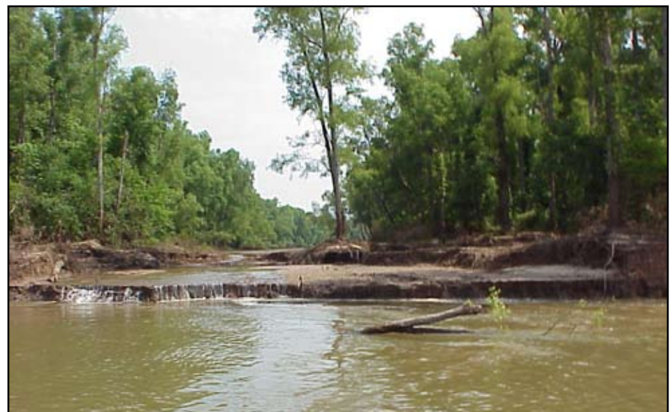
Damaged Arkansas - White Cutoff Structure
