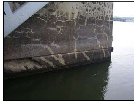
David D. Terry L&D Cracks
