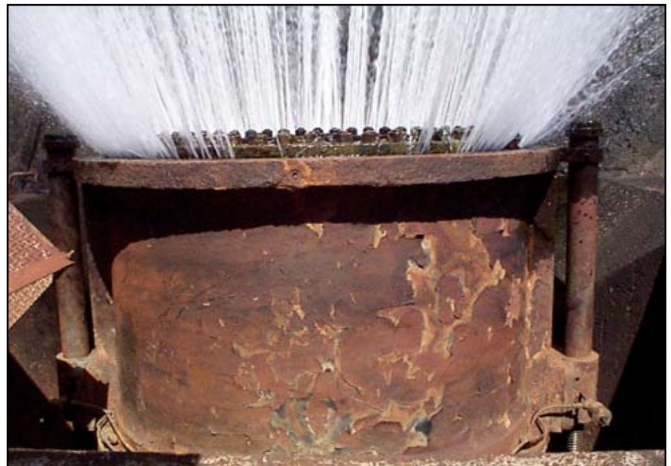
Overhead View of a Nimrod Dam Howell Bunger Valve
