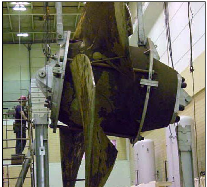
Ozark Powerhouse turbine
