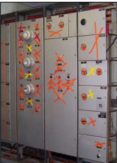
Lock & Dam Control Panel
