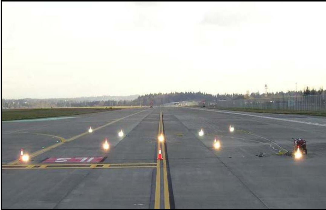
Figure A-20. In-Pavement Lighted X on Taxiway Tango (SEA-TAC)
