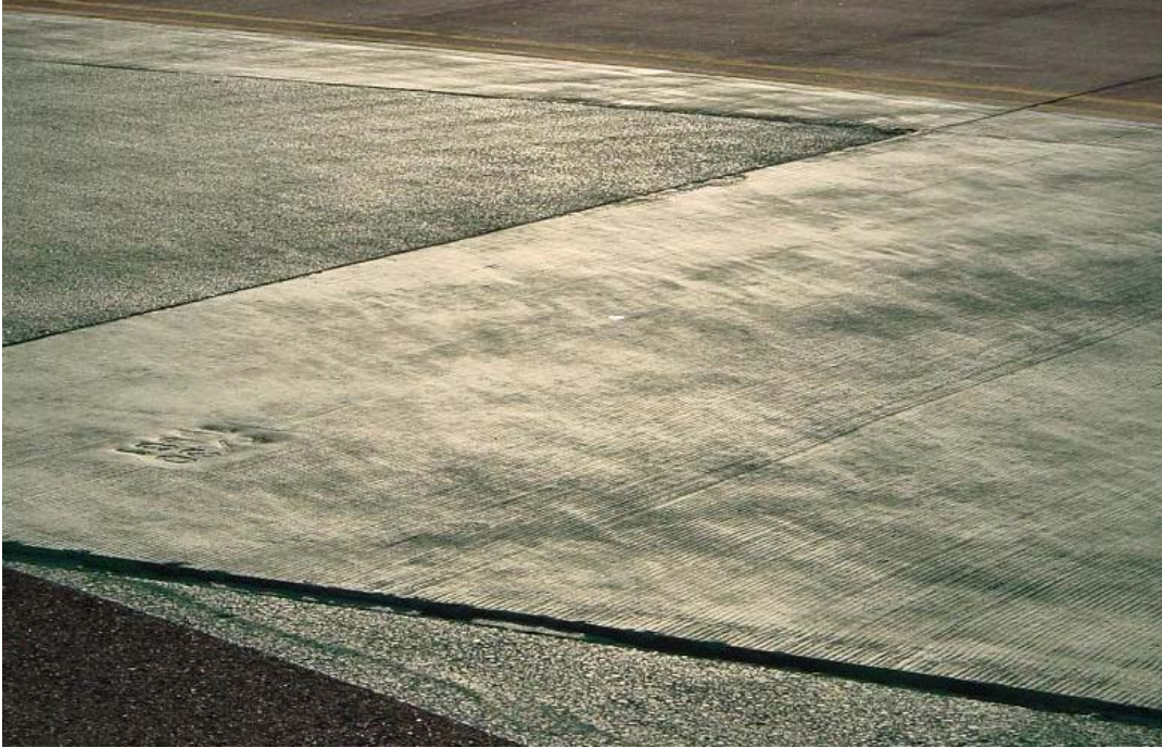
Figure A-3. Sun Glare on Black Surface Treatment (SEA-TAC)
