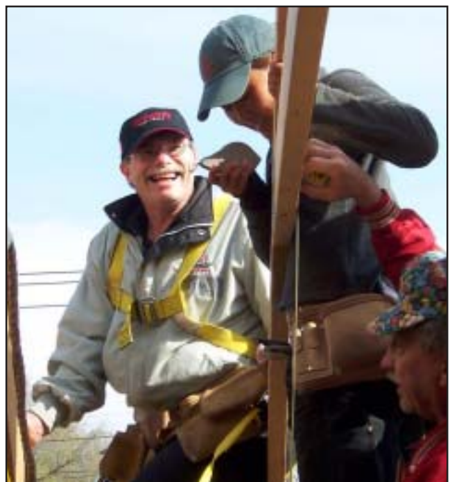
Jim Mosner (left), engineering and construction, works with two volunteers from Habitat for Humanity.
