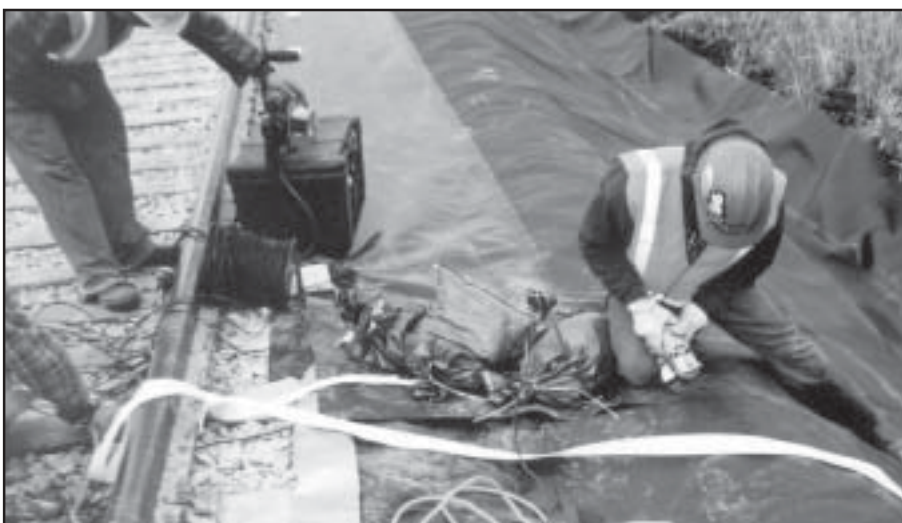
A worker from Arrow-Crete Construction, LLC, of Milwaukee, Wis., grinds seams on the spur-line to prepare for welding them.
