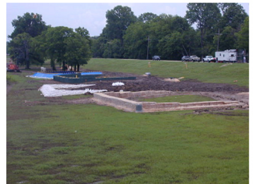
Flood-fighting structures in field test (back to front: Portadam®, HESCO Bastion Concertainer®, sandbags, and RDFW)
