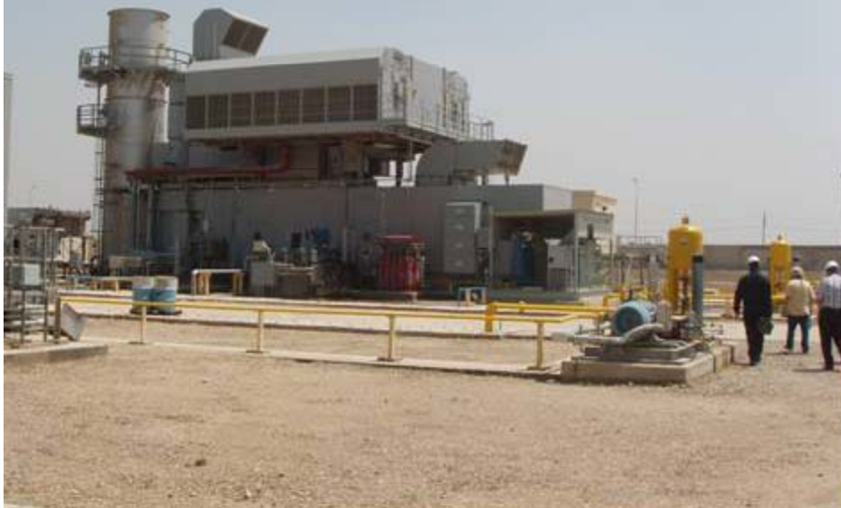
Qudas Power Plant
