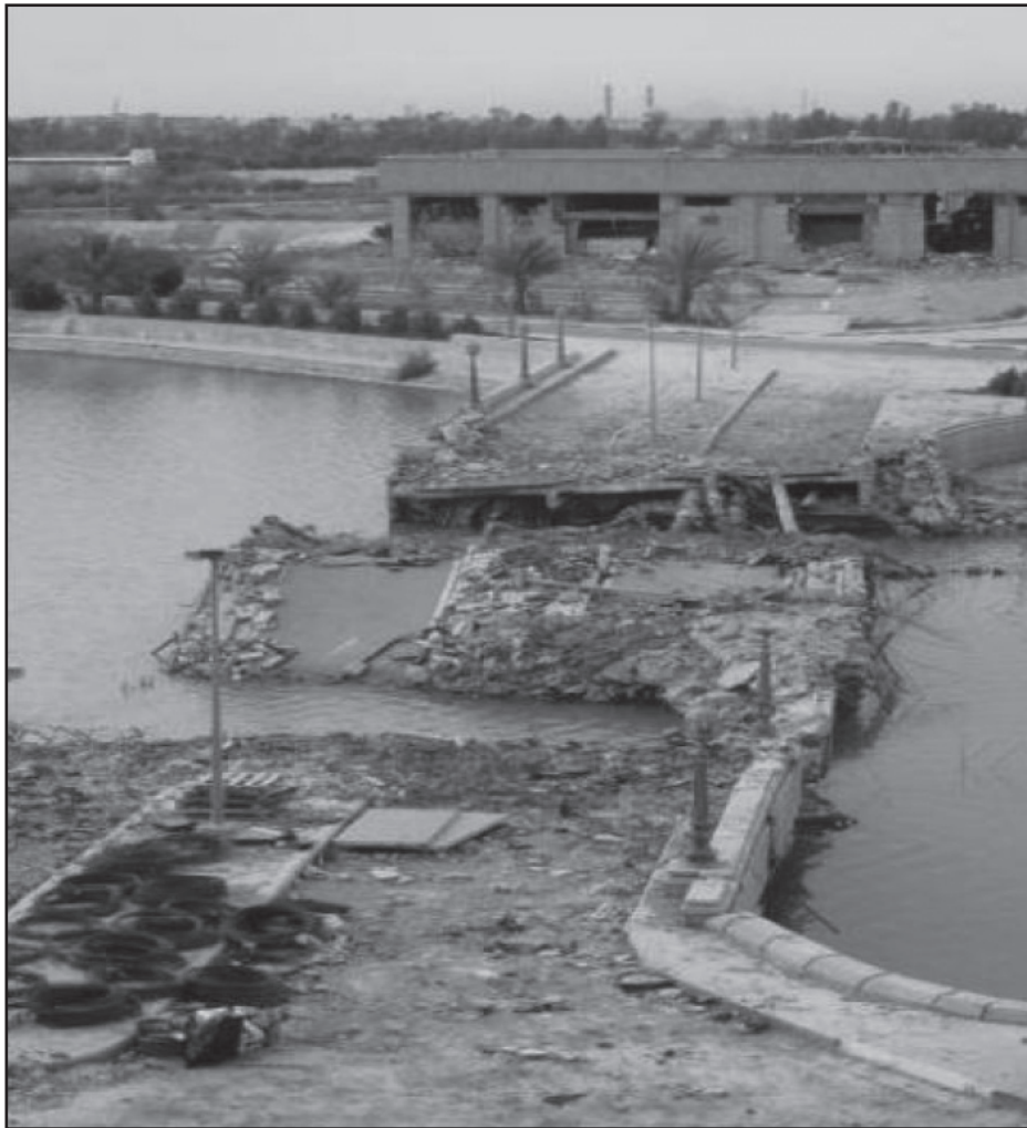
Figure 187. Bomb-damaged bridge, Baghdad
