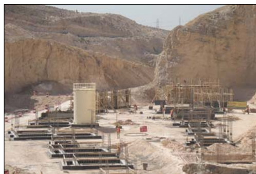
Construction begins on a village at the King Abdullah II Special Operations Training Center in Jordan.
