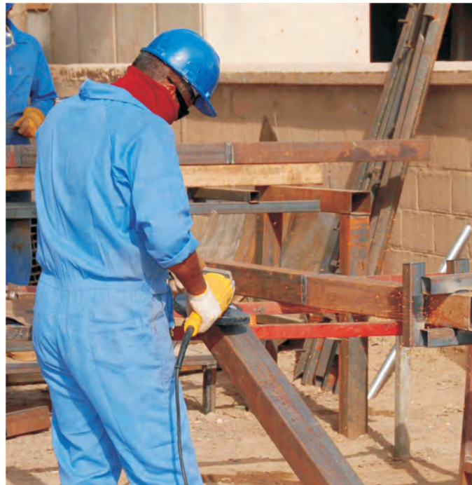
Grinding down the welds on an Anbar Judicial Complex steel fence post produces sparks.
