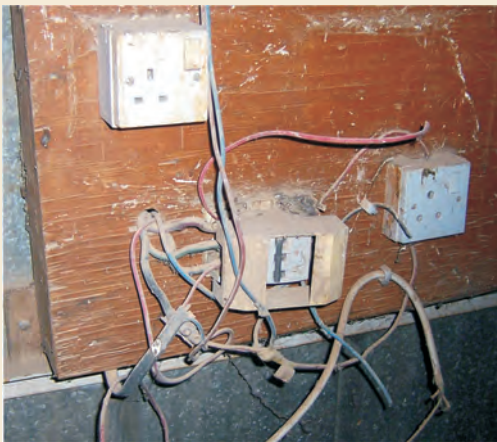
Substandard wiring found by Task Force Safe.
