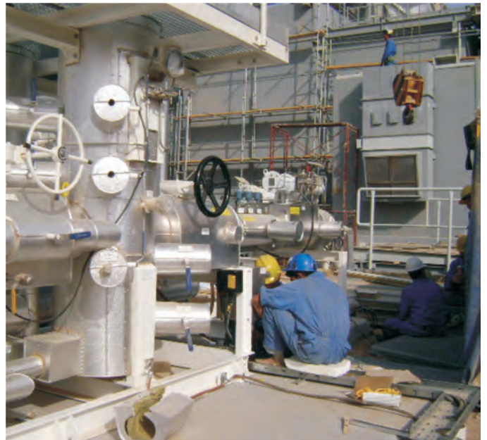
More than 200 Iraqi skilled and semi-skilled laborers are working at the Qudas expansion initiative, which started first in September 2006, and will result in an additional 200 megawatts of power added to the electrical grid.
