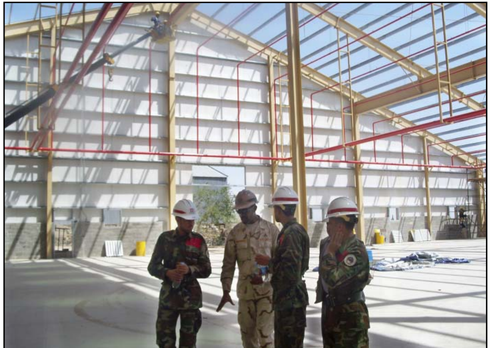
Construction Representative William D. Breckinridge (2nd from left) discusses with the Cadets how the foundation and concrete slab was constructed at a logistics warehouse and how long it took. (Photo by Leslie J. Wright, Capacity Development Program Manager)
