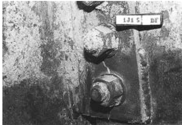
Figure 1-5 Vertical Fracture through Beam Shear Plate Connection
