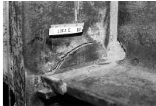
b. Column Flange "Divot" Fracture
