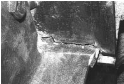
a. Fracture at Fused Zone
