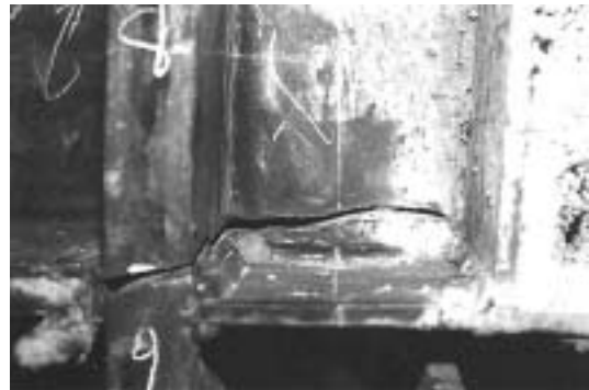
b. Fracture Progresses into Column Web
