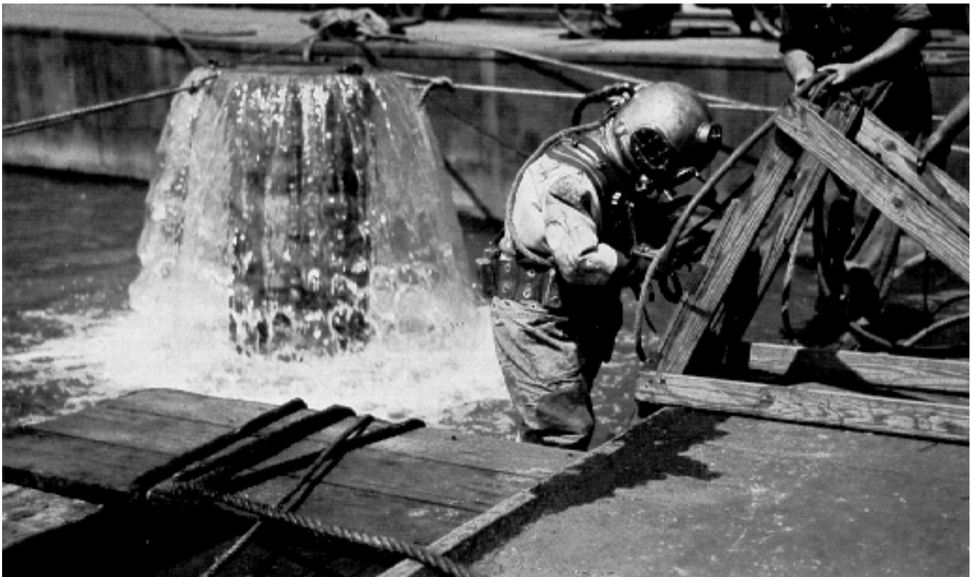
Almost from the beginning, Lock #26 experienced problems. Here a diver descends to investigate a section of the dam where an unusual discharge was indicated.
