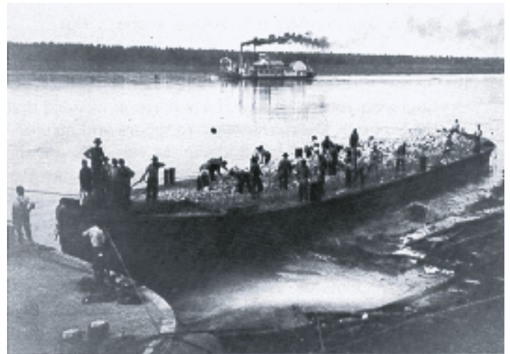
Mattress revetment was sunk into place by the use of large rocks, as shown in the picture.
