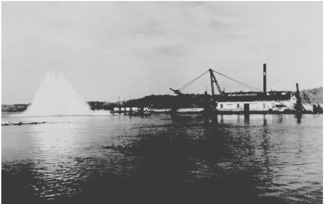
Modern river work includes the use of dynamite to remove rocks as pictured here in the Thebes, Illinois- Commerce, Missouri, area. The dredge Keokuk is seen working at right.
