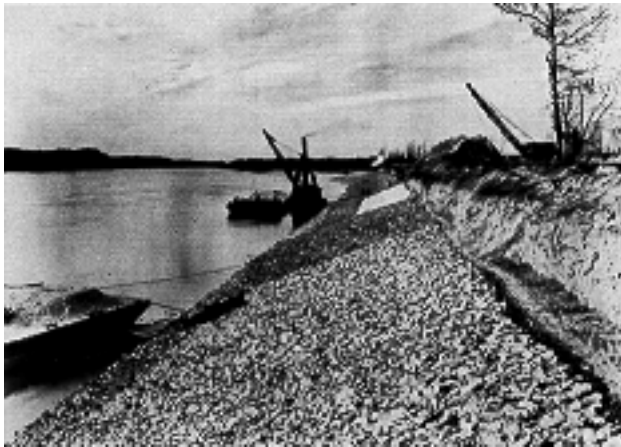
Rip-rap being placed on the banks to prevent erosion. In earlier days, rip-rap was placed by hand.
