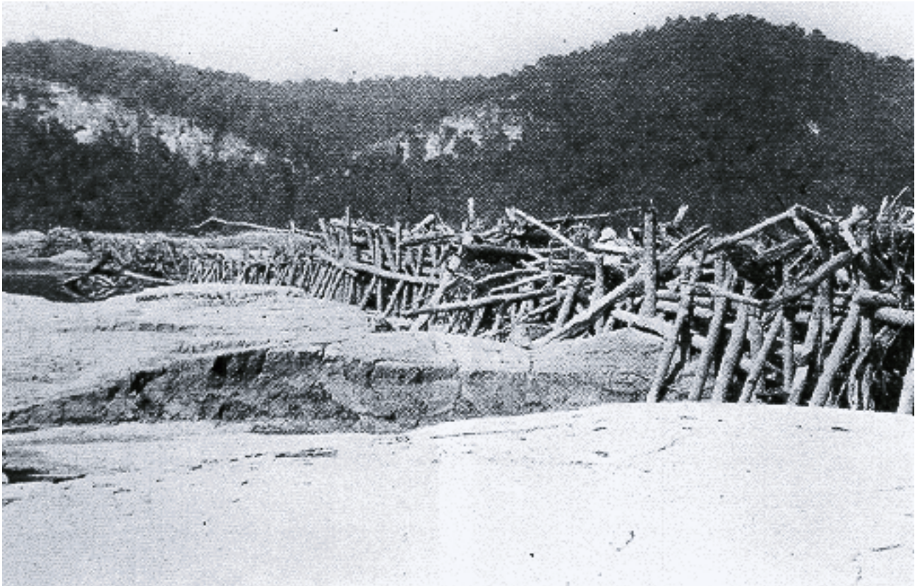
The results of an effective hurdle or piling dike is an accumulation of drift above the hurdle and a deposit of sand below.
