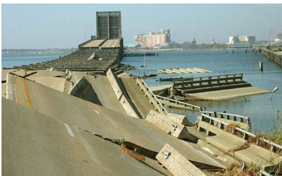
Louisiana Hurricane Katrina U.S. 90 Ocean Springs
