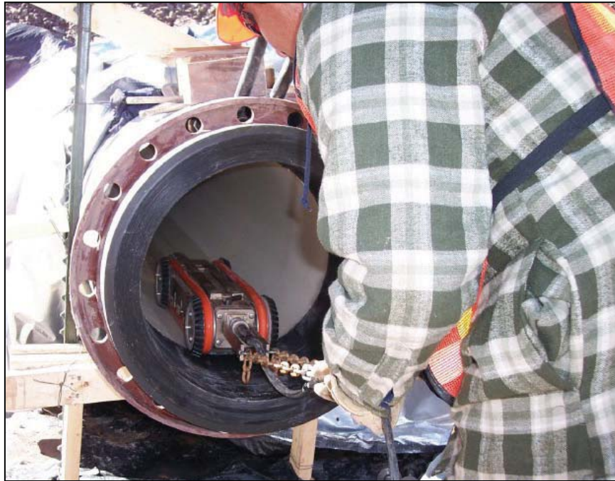
Figure 88. —CCTV inspection of a newly installed slipliner for an outlet works renovation.
