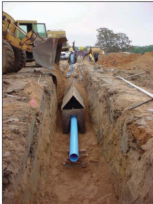
Figure 80. —A trench box or “doghouse” has been used to place material around drainpipes in vertically sided trenches in low hazard potential dams. Vertically sided trenches should not be used in significant and high hazard potential dam construction.
