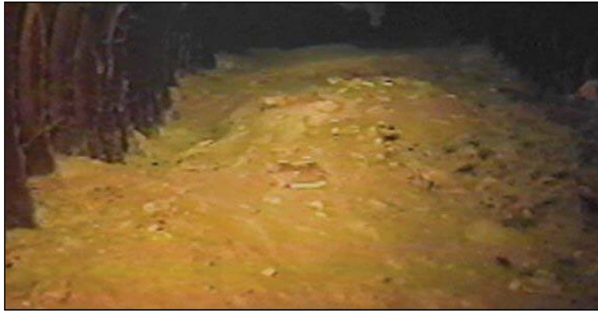
Figure 99. —Sediment deposit on the invert of a HDPE drainpipe.
