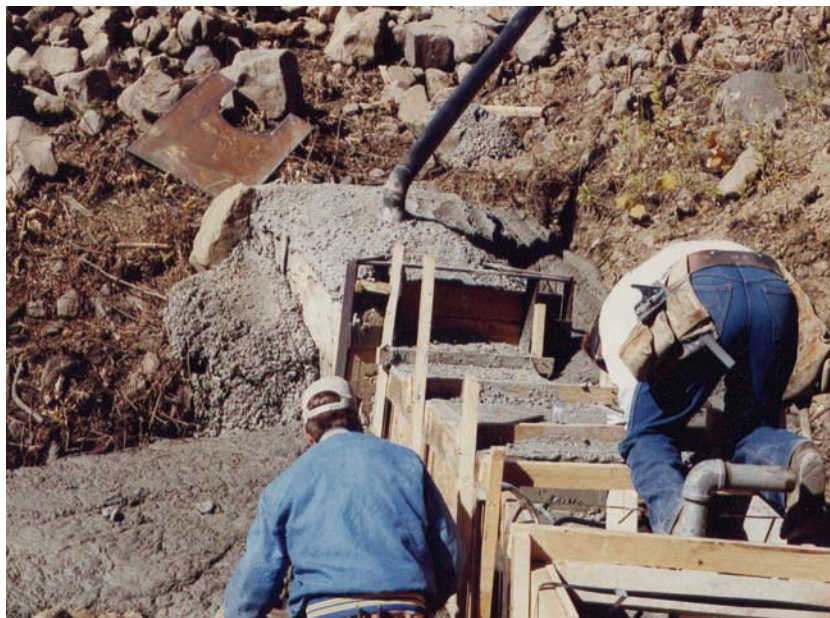
Figure B-16. —Looking upstream towards toe of dam: View of old box conduit and new downstream concrete encasement, during grout operation. Grout pipe is shown in top of photo.
