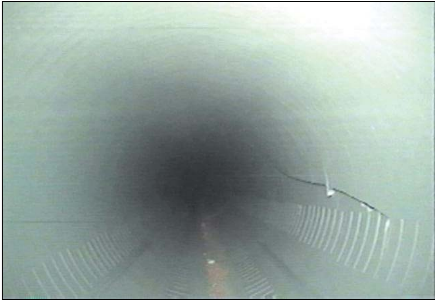
Figure 94. —Slotted PVC pipe used for toe drain has experienced longitudinal cracking. The cracking occurred during construction.
