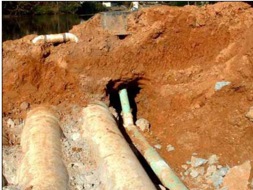
Figure B-13. —After about 10 years of operation, seepage was observed on the downstream slope of the dam in the vicinity of the siphons, and the overlying embankment material was excavated to expose the pipes to determine the source of the seepage.
