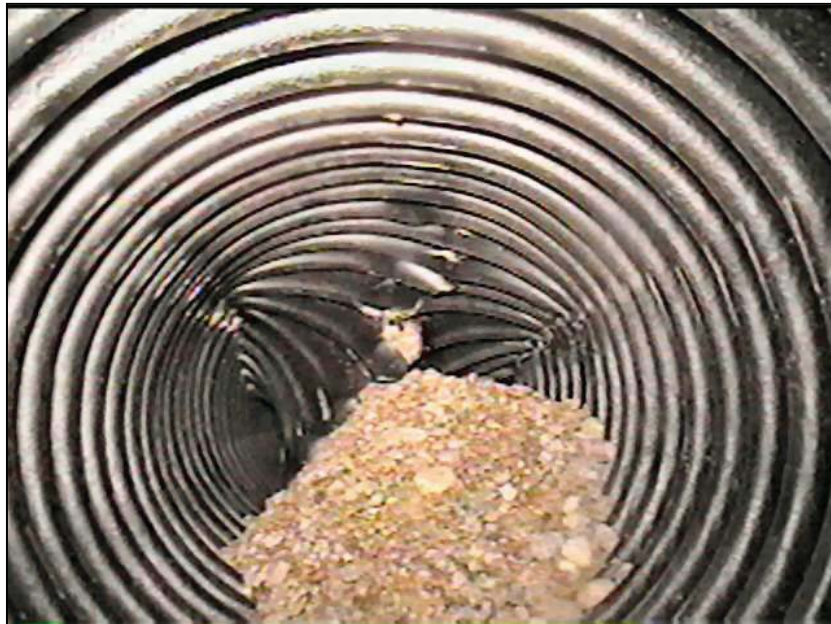
Figure 92. —Single wall corrugated HDPE drainpipe experiencing failure due to buckling.
