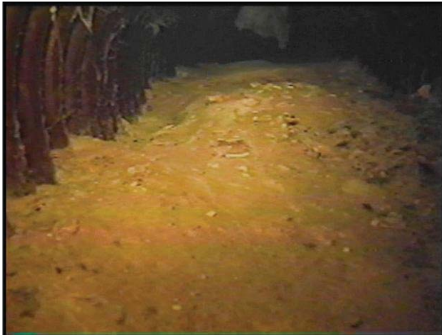
Figure B-2. —The typical amount of sediment deposition observed in toe drain during the November 2000 inspection.
