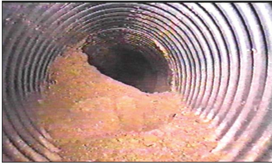
Figure 93. —This HDPE drainpipe has experienced joint separation allowing backfill materials to enter the drainpipe.
