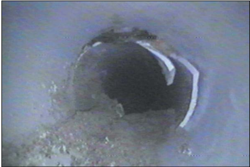
Figure 95. —PVC pipe used for toe drain has experienced transverse cracking. The cracking occurred during construction.
