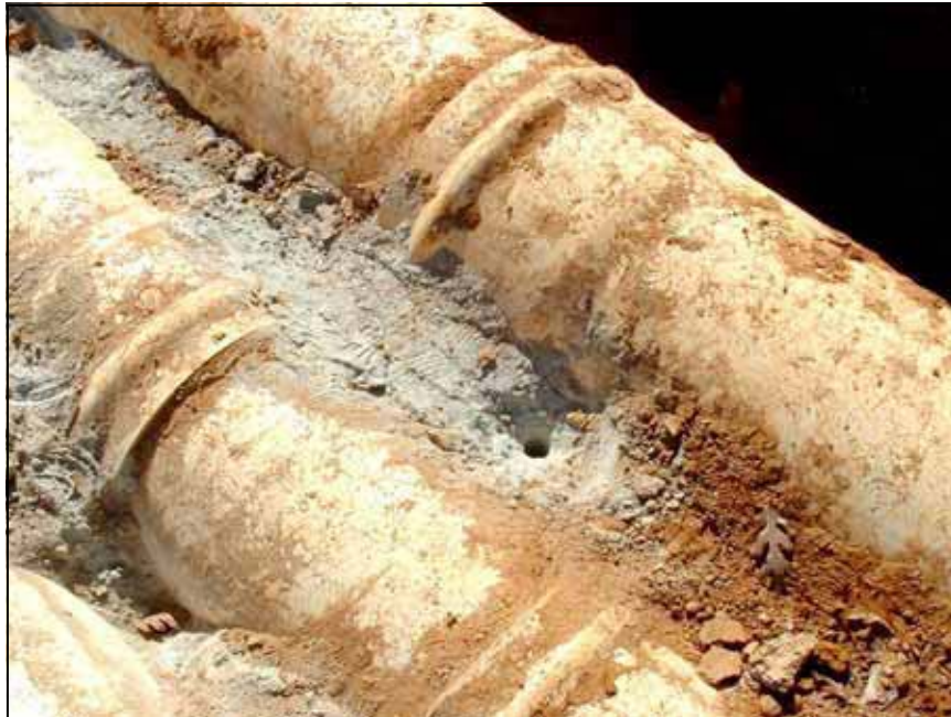
Figure B-14.—A small hole drilled through the concrete bedding between the siphons did not encounter voids under the concrete, even though the designer suspected that seepage was occurring directly under the pipes.
