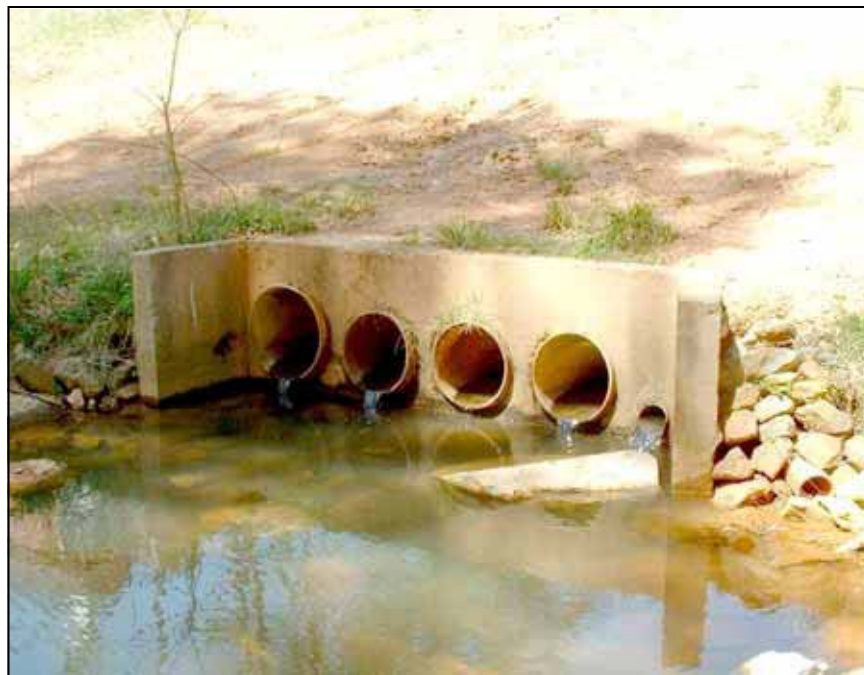
Figure B-12. —In the early 1990's the spillway capacity of the dam was increased by construction of a system of 5 PVC siphons embedded in concrete in a shallow trench through the dam.
