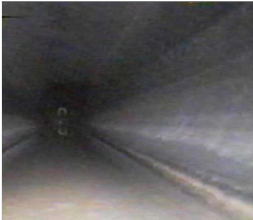
Figure 87. —Looking upstream toward the control gate in an HDPE sliplined outlet works conduit using CCTV inspection equipment.
