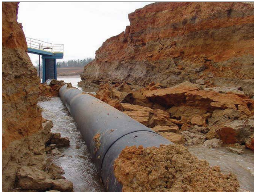
Figure B-9.—Breach showing 36-inch diameter HDPE pipe and riser.
