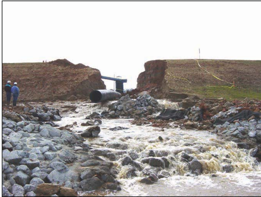
Figure B-8.—Looking upstream through the breach. Embankment was 18 feet high at breach.
