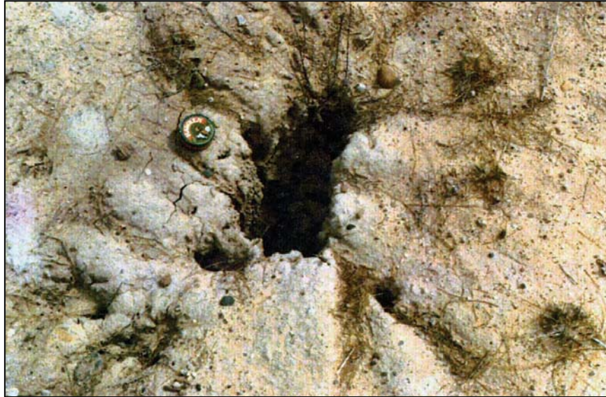
Figure B-4. —Subsurface fissure located at the downstream toe of the dam east of the outlet works. The subsurface soil had a very high moisture content.
