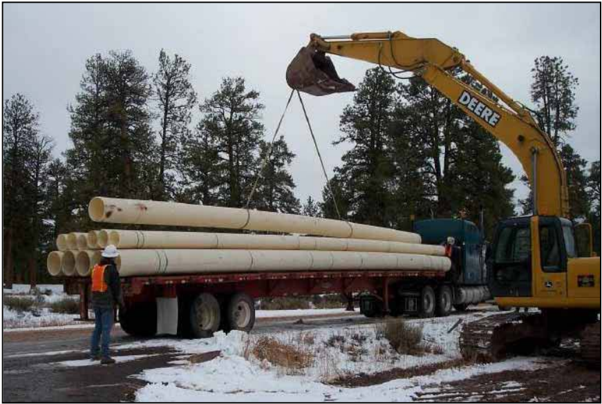
Figure B-23.—HDPE pipe being unloaded at the site using a John Deere 230LC excavator.
