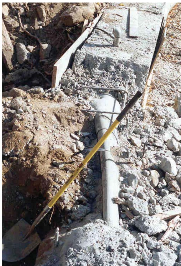
Figure B-17. —Looking downstream from toe of dam after excavation of collapsed portion of HDPE pipe (located in original box conduit, upstream of new concrete encasement).
