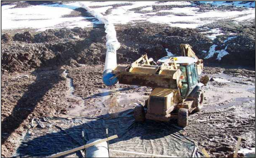
Figure B-24.—Guiding the 20-inch pipe into the upstream end of the CMP.
