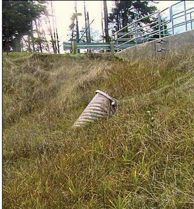
Figure 90. —Cleanout provides access to the drainpipe for CCTV inspection.
