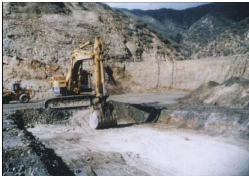
Figure 85. —Contaminated materials being excavated beneath a roadway crossing over a filter. Photo courtesy of ASDSO (Hammer, 2003).
