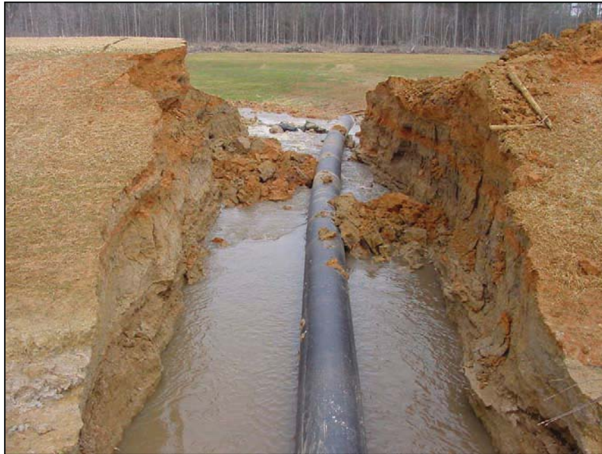
Figure B-10. —View looking downstream along the pipe. The breach was 26 feet wide.
