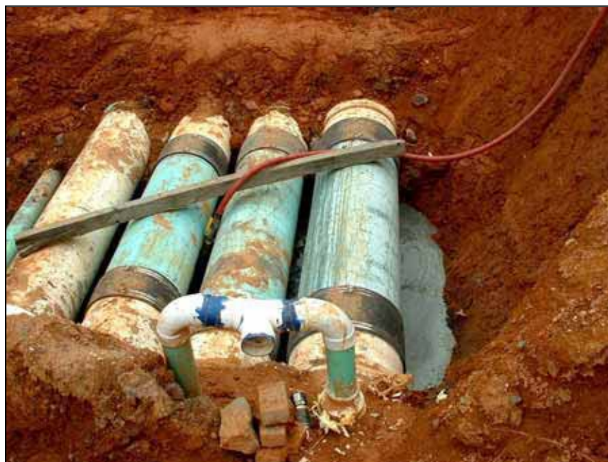
Figure B-15.—After removal of portions of the PVC siphons, it was determined that the original concrete bedding had been improperly placed, resulting in voids under the centers of the pipes. Portions of the siphons were replaced, and the bedding was replaced with a high slump concrete.
