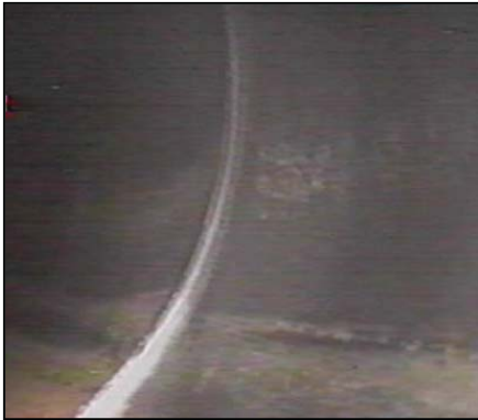
Figure 86. —A butt fused, solid walled HDPE pipe joint in an outlet works slipliner as viewed using CCTV inspection equipment.
