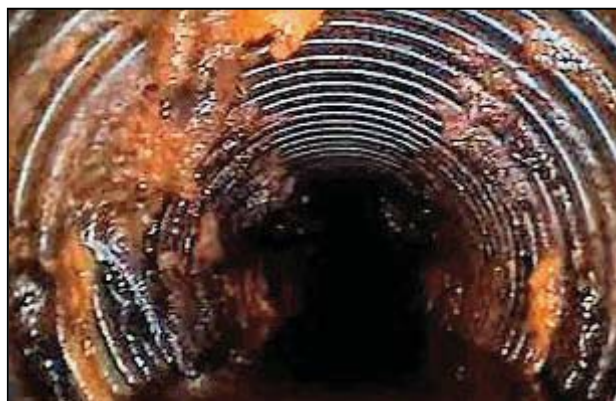
Figure 98. —Iron bacteria have partially blocked the perforations in this HDPE drainpipe. Note that the only open perforation passing seepage is in the lower left corner of figure.
