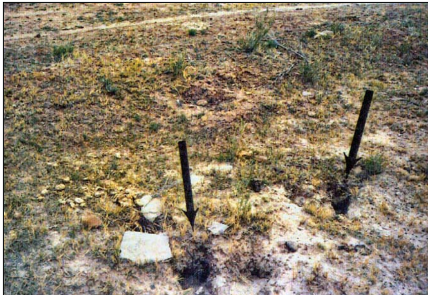
Figure B-5. —Erosional features typically associated with dispersive soils as seen at Ganado Dam. The common name for such features is “jughole.”
