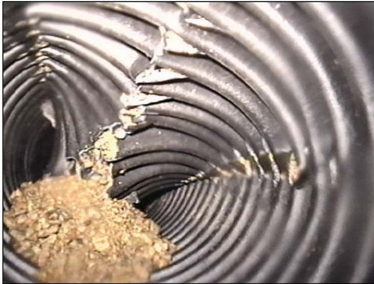
Figure 45. —Single wall corrugated HDPE drainpipe experiencing failure due to buckling.
