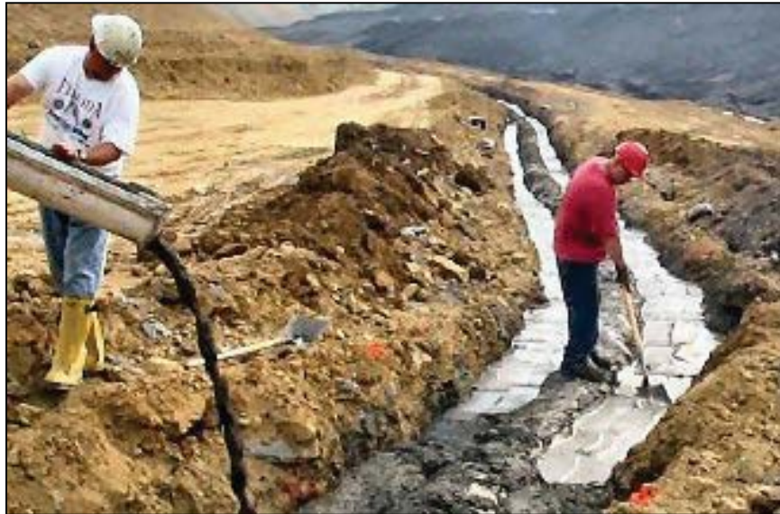
Figure 51. —The CLSM is typically transported to the construction site in ready mix concrete trucks. In this figure, CLSM is being used as a pipe encasement. CLSM should not be used for embankment conduits in significant and high hazard potential dams.
