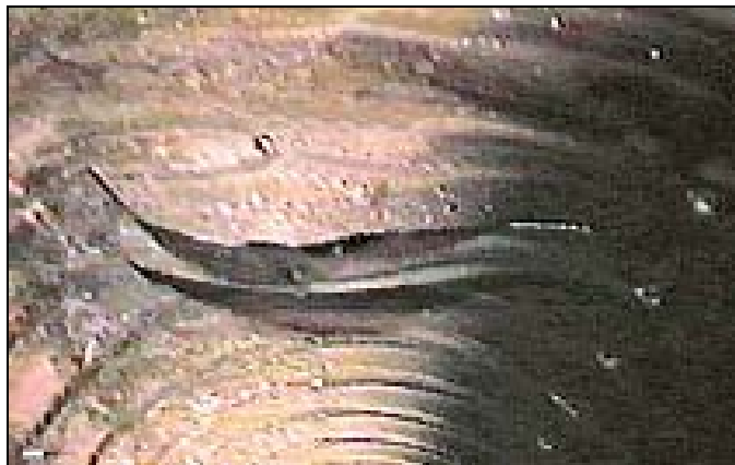
Figure 40. —The crown of this single wall corrugated HDPE pipe has been damaged due to construction traffic crossing over it. Insufficient cover over the pipe was the likely cause.
