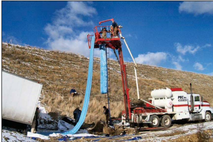
Figure 22. —Contractor installing a resin-soaked CIPP liner into an existing outlet works. Installation begins by hauling the liner up to the top of the platform. On the platform, water is run into the liner causing it to pressurize and expand downward. As the liner reaches the outlet works pipe opening, laborers on the ground maneuver the water filled liner into the outlet works. Water pressure continues to cause the liner to advance upstream in the outlet works pipe and un-invert itself. Photo courtesy of Tetra Tech Inc.
