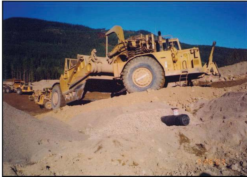
Figure 65. —Construction equipment can travel safely over plastic pipe when adequate cover above the drainpipe is provided.
