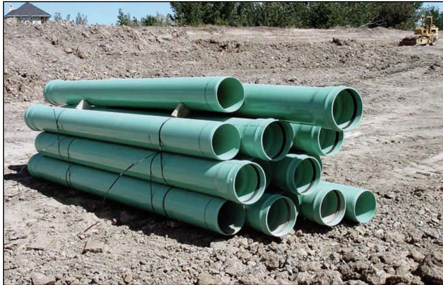
Figure 15. —Solid wall PVC pipe has occasionally been used in embankment conduit applications within low hazard potential embankment dams. However, the bell and spigot joint connection used for this type of pipe can experience separation and seepage when improperly installed.
