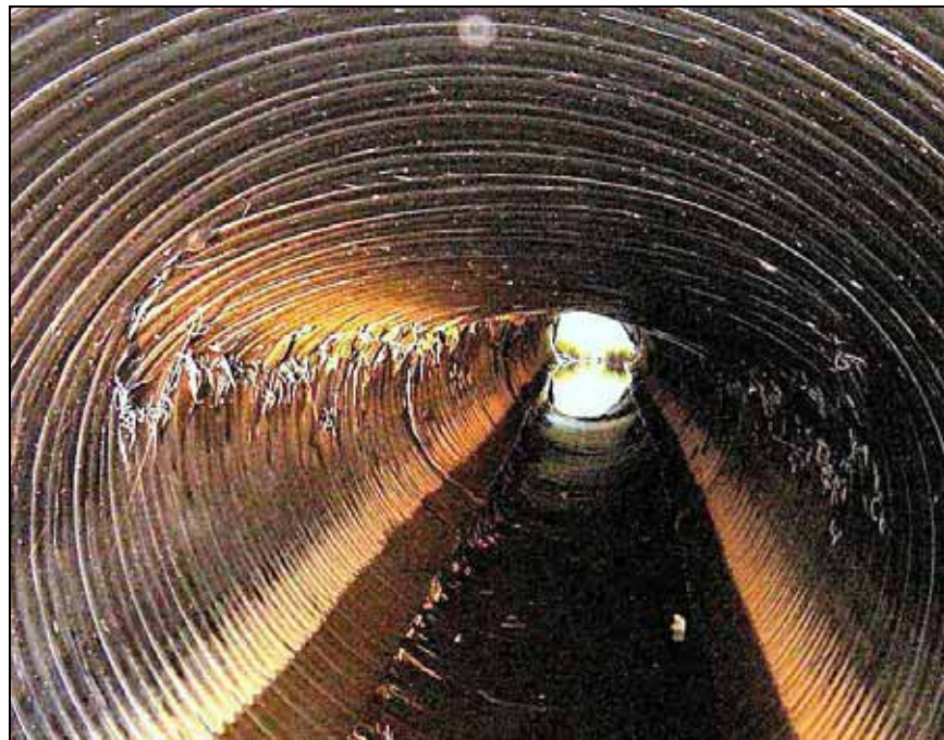
Figure 44.—Single wall corrugated HDPE pipe experiencing wall crushing.
