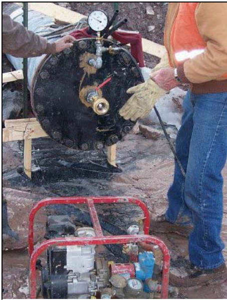
Figure 52. —Leak test being performed on an HDPE slipliner for an outlet works renovation.
