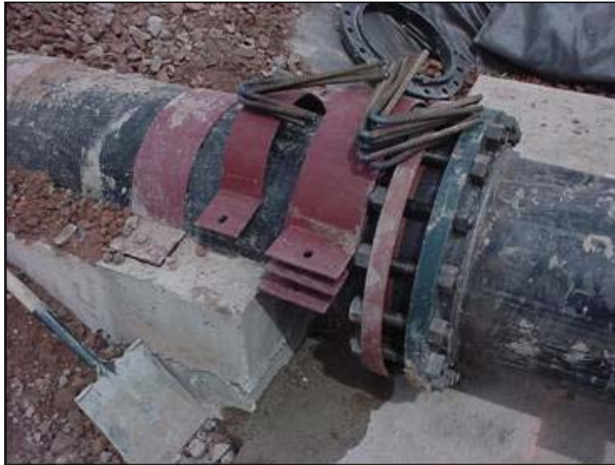
Figure 50. — Until further research is completed, concrete cradles beneath plastic pipe should not be used.
