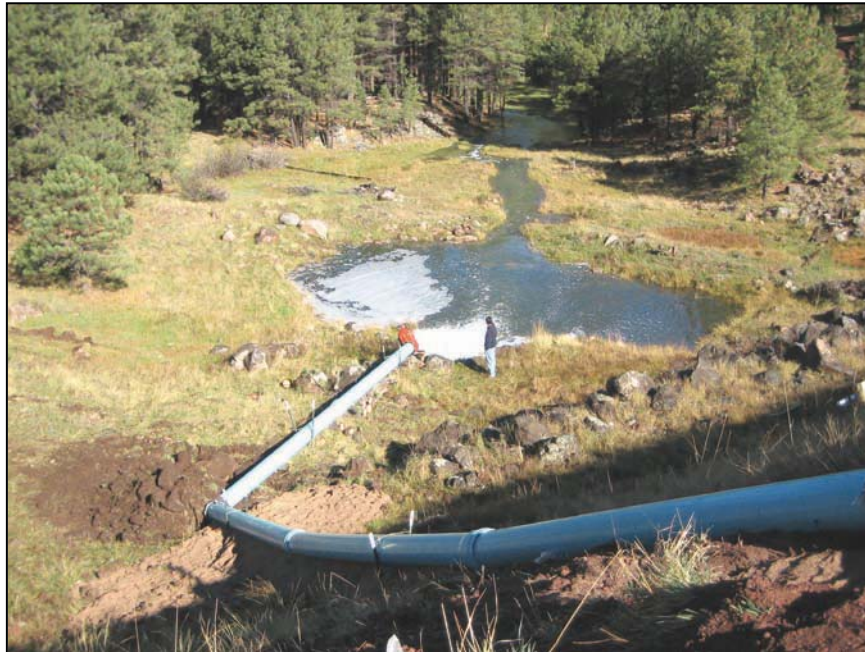
Figure 25. —A temporary siphon constructed using PVC pipe. This siphon is being used for short term operation.
