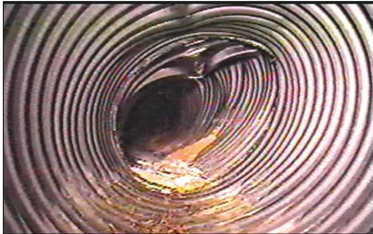
Figure 46. —Single wall corrugated HDPE drainpipe experiencing excessive deflection leading to buckling.
