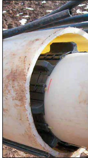
Figure 6. —Dual-wall containment HDPE pipe. A 14-inch diameter carrier pipe is being inserted into a 20-inch diameter containment pipe. Intermediate spacers are attached to the carrier pipe. Grout lines for grouting of the annulus between the existing conduit and containment pipe can be seen.
