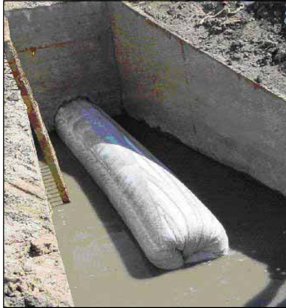
Figure 21. —CIPP liner exiting from an existing outlet works conduit, via the hydrostatic inversion method.
