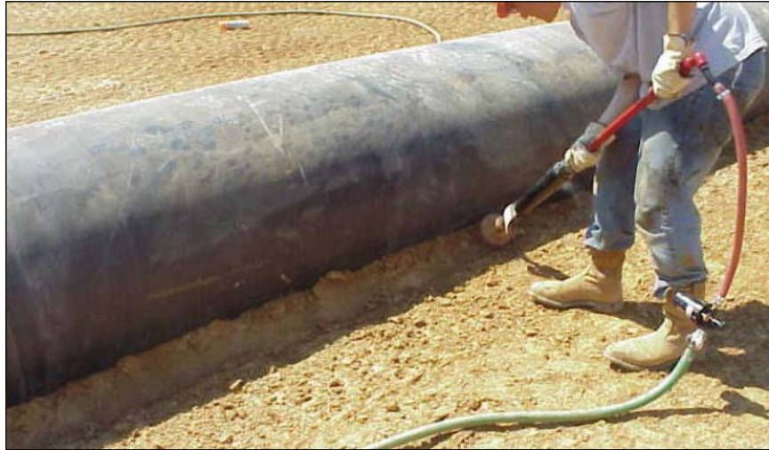
Figure 49. —Compacting earthfill under the haunches of plastic pipe is very difficult and quality compaction can not be achieved.
