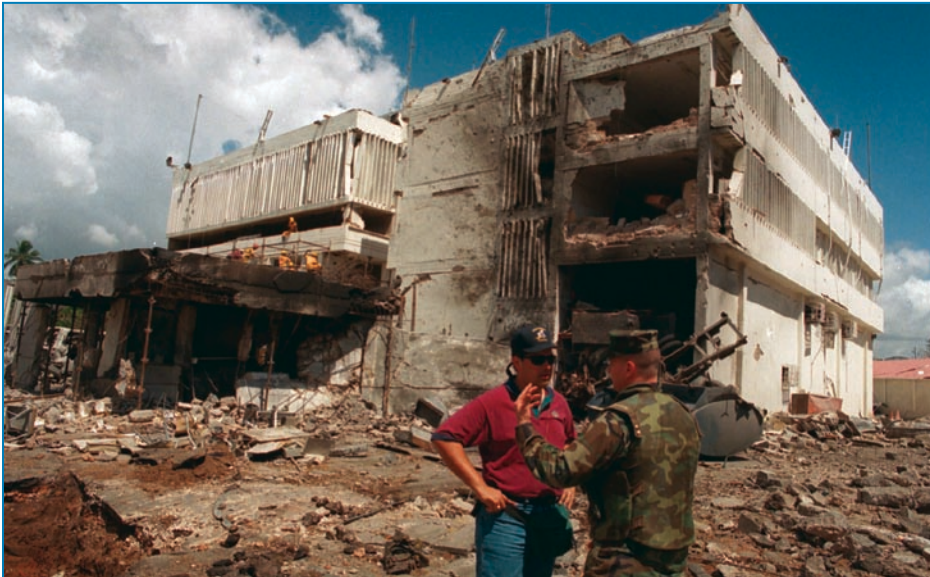
Figure 1-17: Damage to the U.S Embassy, Tanzania
