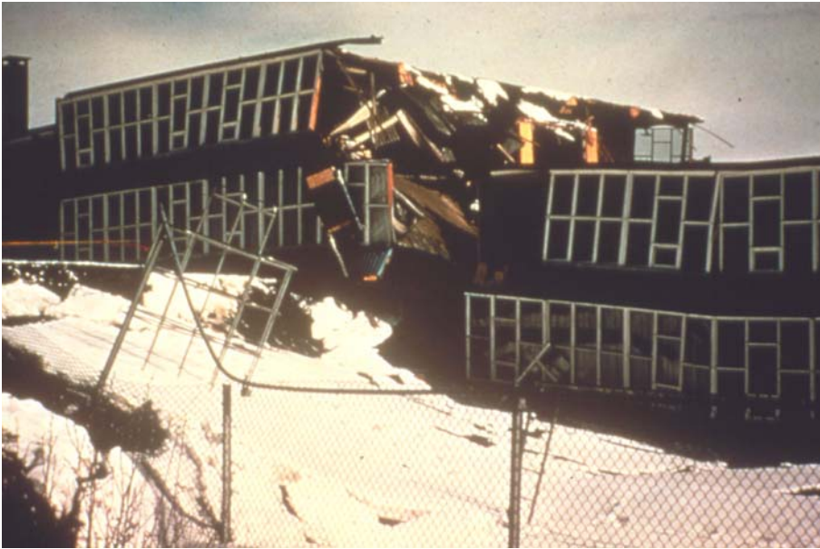
Figure 3-10 Government Hill School, Anchorage, destroyed by landslide during the magnitude-8.4 Alaska earthquake of 1964. (Photo courtesy of National Oceanic and Atmospheric Administration, National Data Service).
