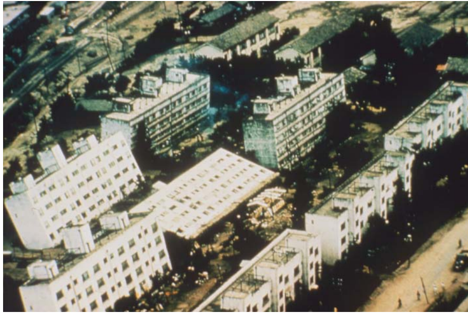
Figure 3-9 Aerial view of leaning apartment houses resulting from soil liquefaction and the behavior of liquefiable soil foundations, Niigata, Japan, earthquake of June 16, 1964. (Photo courtesy of National Oceanic and Atmospheric Administration, National Data Service).
