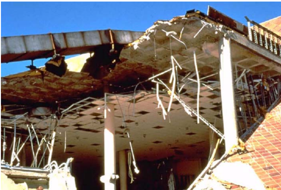
Figure 7-1 Severe damage to a department store severely shaken by the 1994 Northridge earthquake. Shear failure between the waffle slabs and columns caused the collapse of several floors. (photo courtesy of the Earthquake Engineering Research Institute.)
