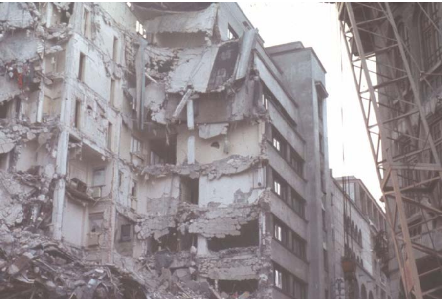
Figure 3-4 Preseismic-code ten-story reinforced-concrete-frame building in Bucharest, Romania, that partially collapsed during the 1977 magnitude-7.2 earthquake approximately 65 miles north of Bucharest. (photo courtesy of C. Rojahn)
