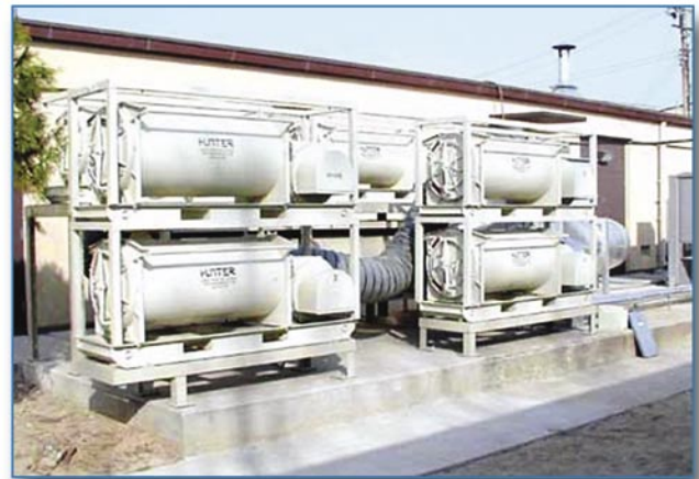
Figure 5-11 A military FFA 580 air filtration system containing both a HEPA filter and an ASZM-TEDA carbon adsorber as part of an overpressure system
