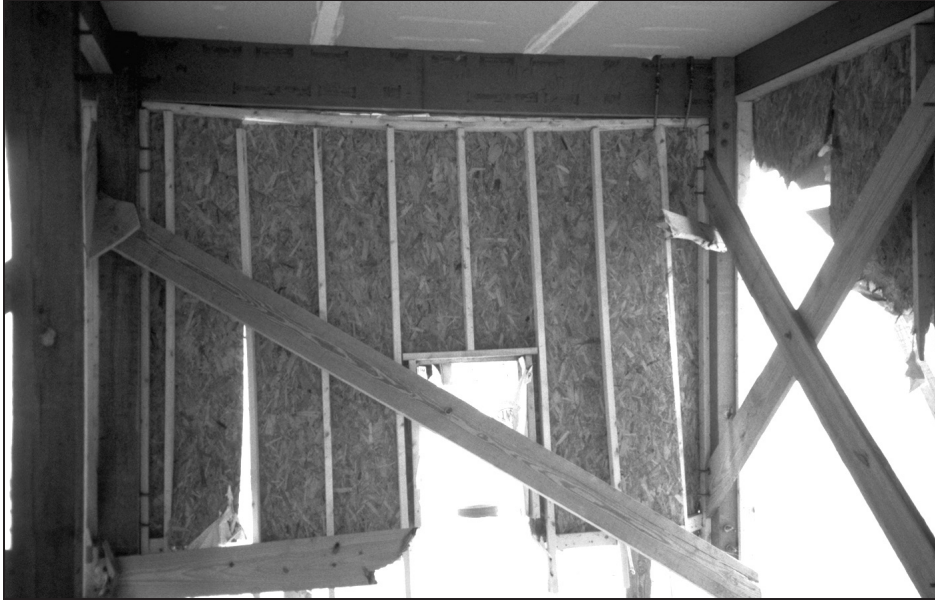
Figure 7. Non-compliant bracing arrangement
