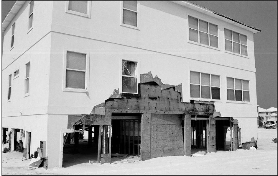
Figure 5. Non-compliant breakaway wall joint detailing
