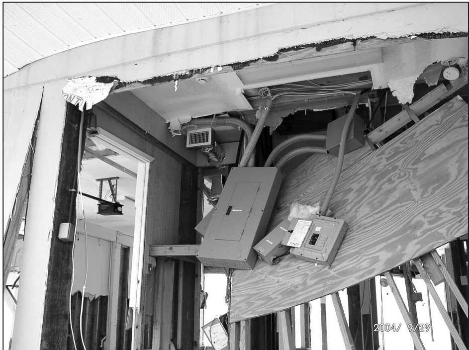
Figure 6. Non-compliant utilities attached to breakaway wall
