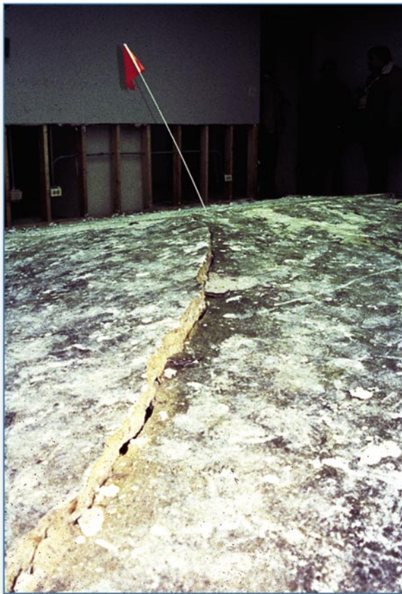
Figure 5-8 Fractured concrete basement floor, Gurnee, IL, 1986
