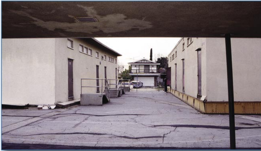
Figure 4-9 Modular classrooms pushed off their foundations; note stairs at left, Northridge, CA, 1994.
