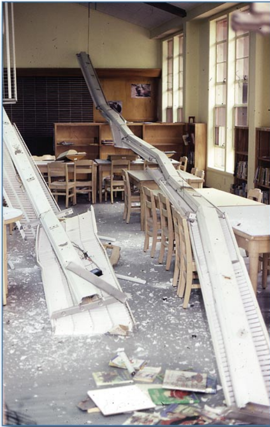
Figure 4-12 Fallen light fixtures, library, Coalinga, CA, 1983 SOURCE: GARY MCGAVIN, REDLANDS, CA
