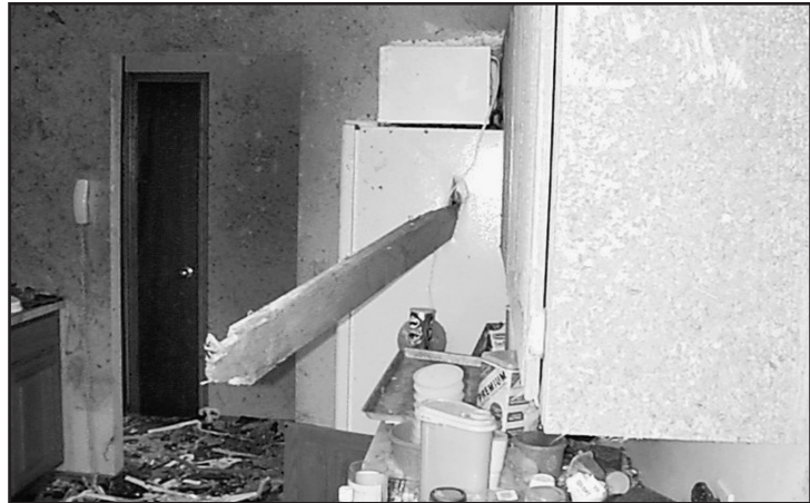
2x6 missile penetrating a refrigerator, Midwest tornadoes of May 3, 1999
