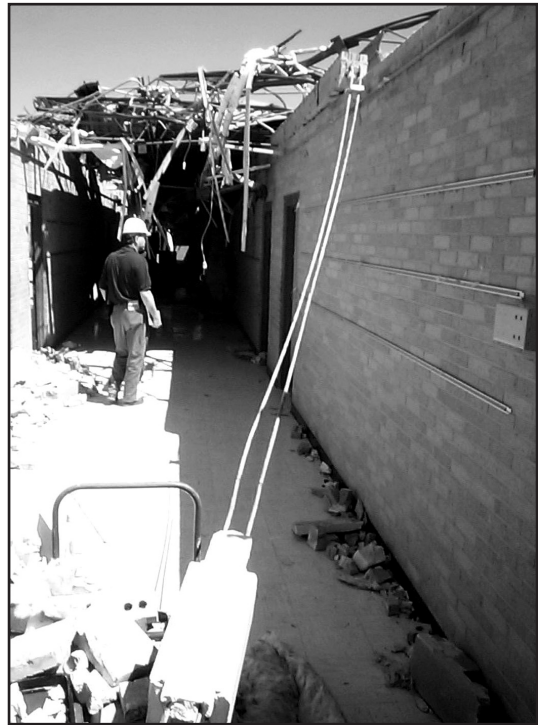
Figure 6-5. Failure in this load path occurred between the bond beam and the top of the unreinforced masonry wall. This school building was in the path of an F4 tornado vortex.
