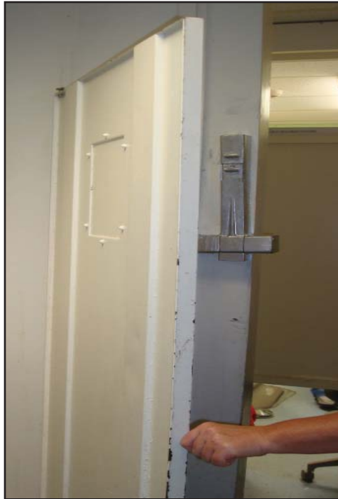
X-Ray staff are exposed to elevated levels of radiation because the walls do not have lead in them. Only a thin door encloses the X-Ray area.
