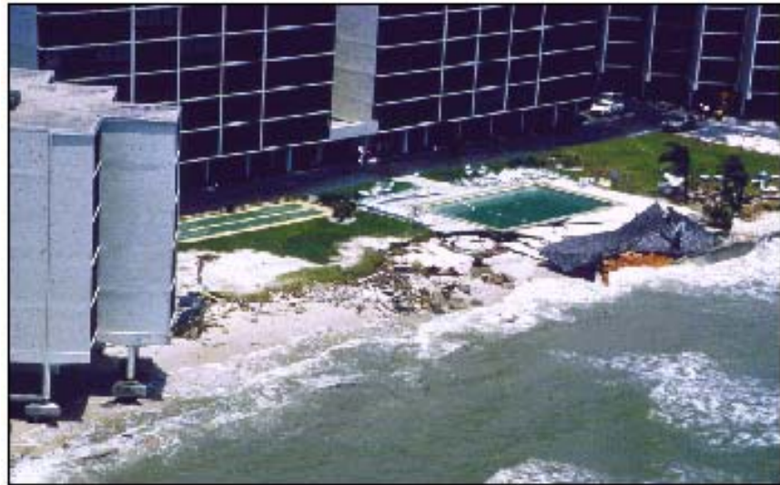
Figure 8-19. Damage at Bonita Beach, FL, from 1982 subtropical storm. Had this building not been supported by an adequate pile foundation, it would have collapsed.
