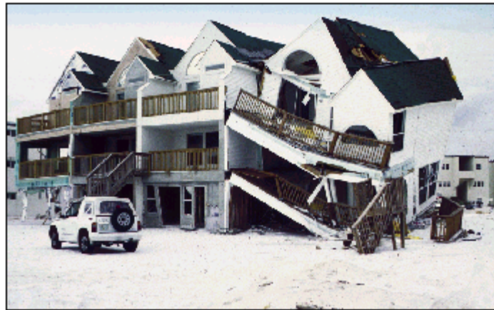
Figure 8-1. Hurricane Opal (1995). Damage to new construction in a mapped A zone. The flood and debris damage could have been avoided had the site been considered a coastal A zone and had the structure been elevated on an open foundation.
