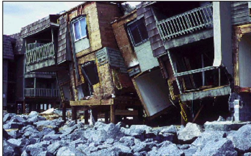
Figure 8-18. Damage to buildings sited close to an eroding shoreline. Garden City Beach, SC, Hurricane Hugo (1989). Storm waves often overtop revetments and damage buildings.
