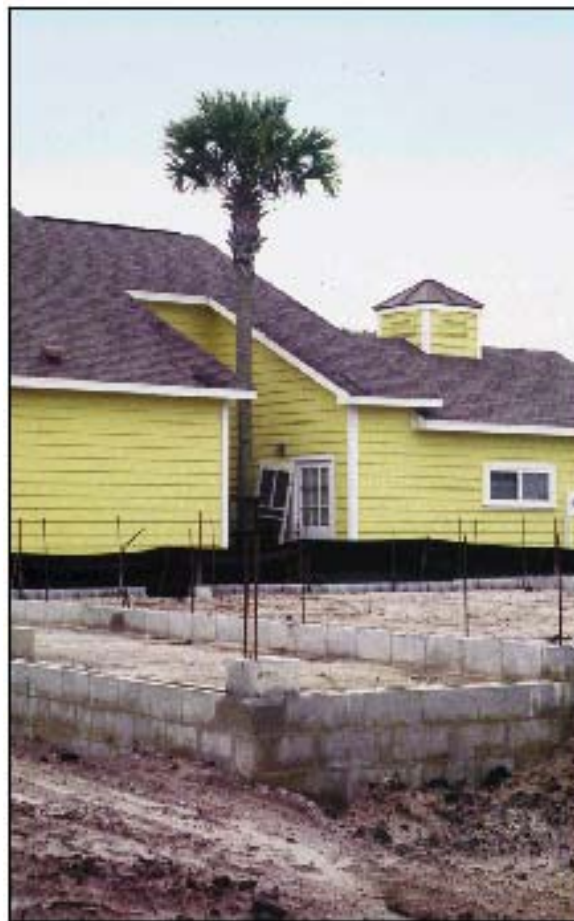
Figure 8-20. Avoid notching for trees. Siting and designing buildings to accommodate large trees is important for a variety of reasons. However, notching the building and roofline to allow placement around a tree can lead to roof and envelope damage during a high-wind event.
