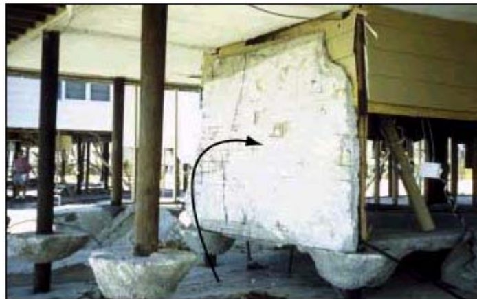
Figure 6-12. Hurricane Fran (1996). Concrete slab-on-grade flipped up by wave action came to rest against two foundation members, generating large unanticipated loads on the foundation.
