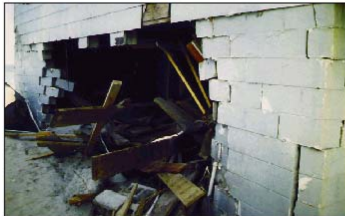
Figure 6-14. Hurricane Fran (1996). Debris lodged beneath a Topsail Island, NC, house elevated on unreinforced masonry walls. The wall damage could have resulted from flood and wave forces, debris loads, or both.
