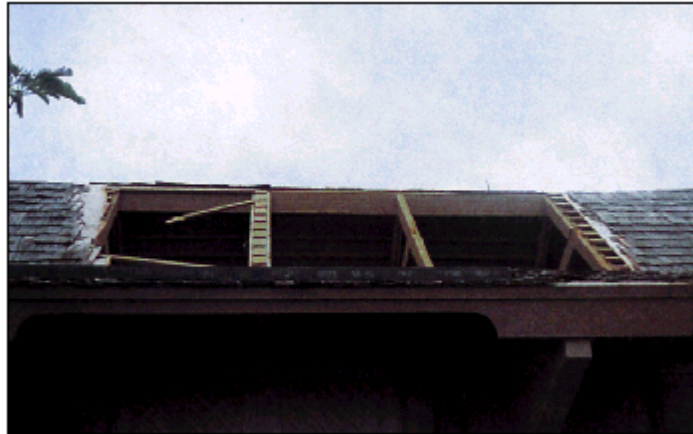
Figure 6-18. Hurricane Iniki (1992), Kauai County, Hawaii. Loss of roof sheathing from improper nailing design and schedule.
