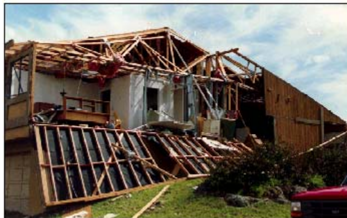
Figure 6-17. Hurricane Andrew (1992). End-wall failure of typical first-floor masonry/second-floor wood-frame building in Dade County, Florida.
