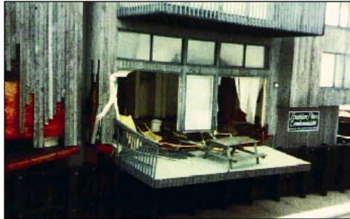
Figure 6-11. Damage to an oceanfront condominium in Ocean City, NJ, caused by wave runup on a timber bulkhead.
