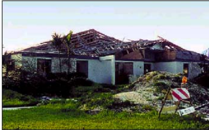
Figure 1-7. Hurricane Andrew (1992). Roof structure failure from inadequate bracing.
