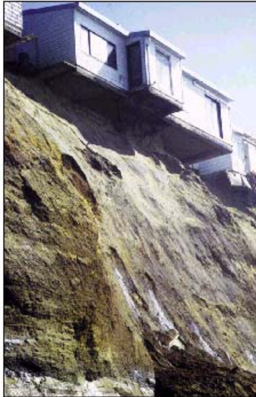
Figure 1-12. Winter Coastal storms, California and Oregon (1997–1998). House in Pacifica, CA, undermined by bluff erosion.
