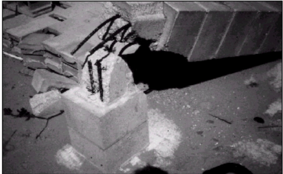
Figure 1-5. Hurricane Hugo (1989), South Carolina. Failure of reinforced masonry column.
