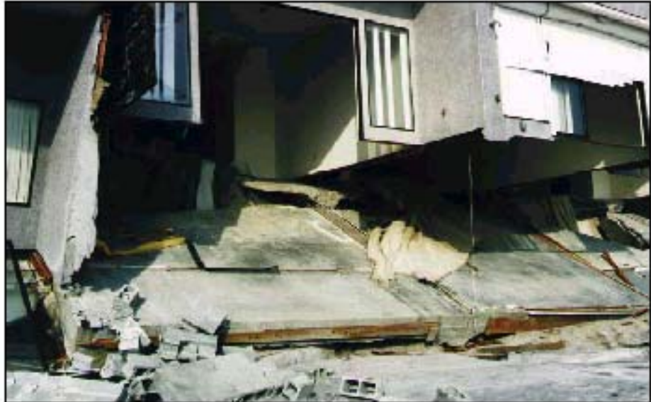
Figure 1-11. Hurricane Opal (1995), Bay County, Florida. Building damage from erosion and undermining.
