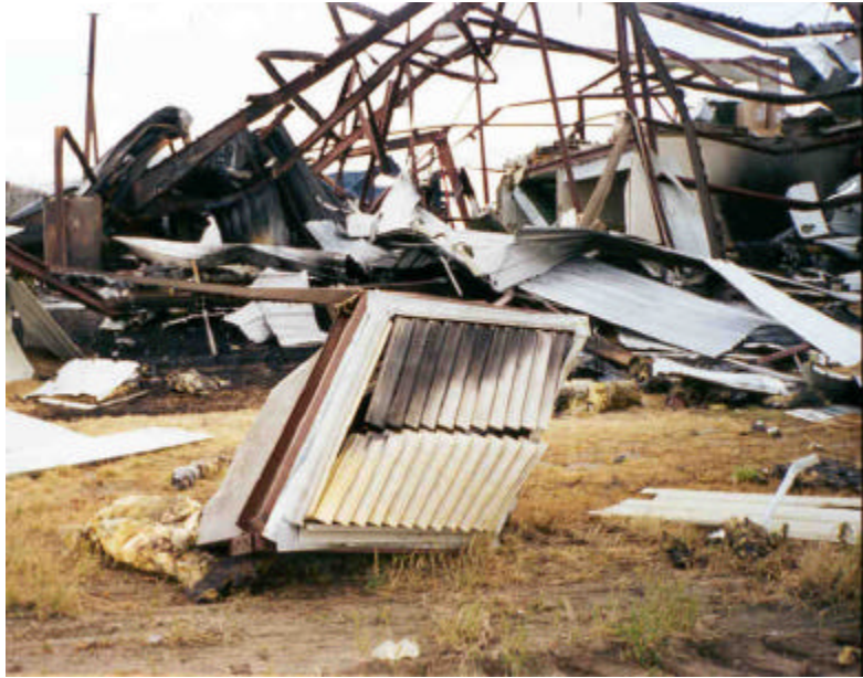
Figure 8. Ventilation Fan with Yellow Residue
