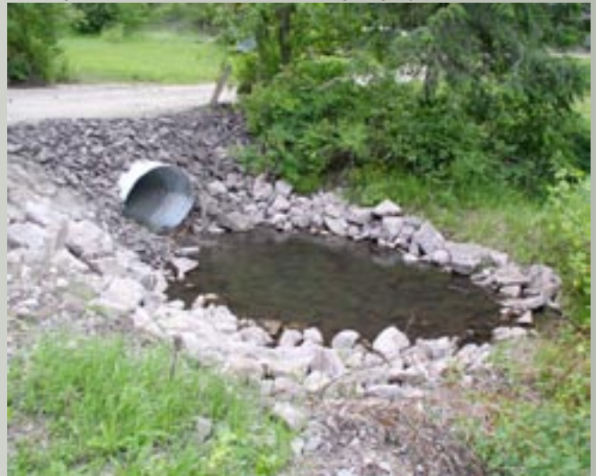
The outlet areas of the culverts were armored so that the roads would not erode. The areas disturbed have been seeded with slender wheatgrass.
