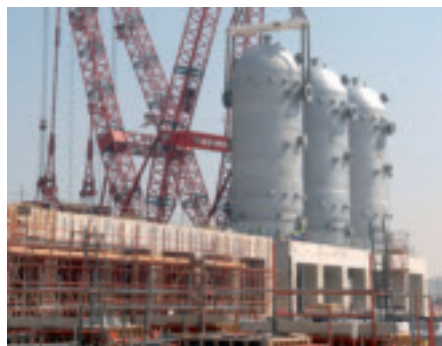
HPS reactors at Pearl GTL
