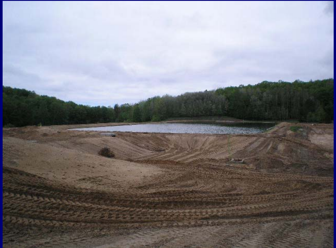
The Village of Honor's Lagoon Sewage Treatment System
