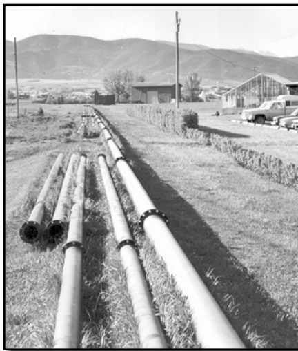
Construction of a 2,000-foot hydraulic chip pipeline at Bozeman for cooperative studies by the Station and Montana State was near the halfway point in this photo.
