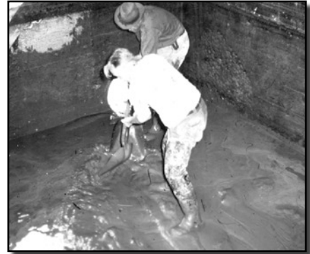
Perry Plummer (foreground) grabbed a shovel and helped technician Paul Hansen clear out a sediment tank after heavy summer storms at Great Basin (about 1940).
