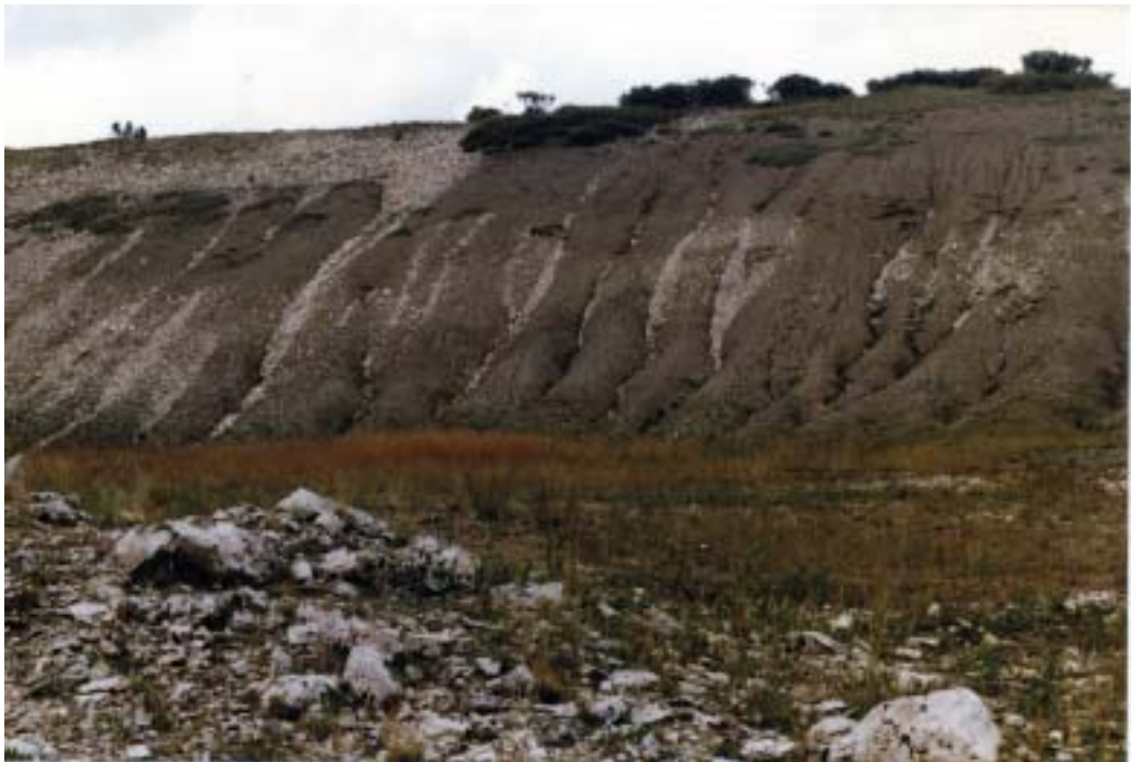
Figure 39—Site F, August 30, 1990 (detail) —Note the continued cutting of slopes by water as evidenced by exposed white rock fragments. Upper portion of the slope appears to have lost 8 to 9 inches of soil since 1972. Shrubs are trying to establish on the eroded areas.
