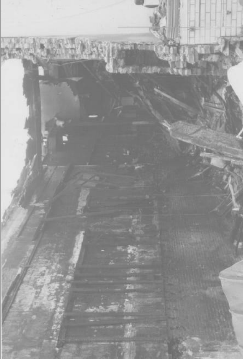
Photo by Ty Dickerson Void in brick wall (foreground) was a flue from a heating unit (previously removed) that may have allowed smoke from the basement to vent to the outside in the early stages of the fire.
