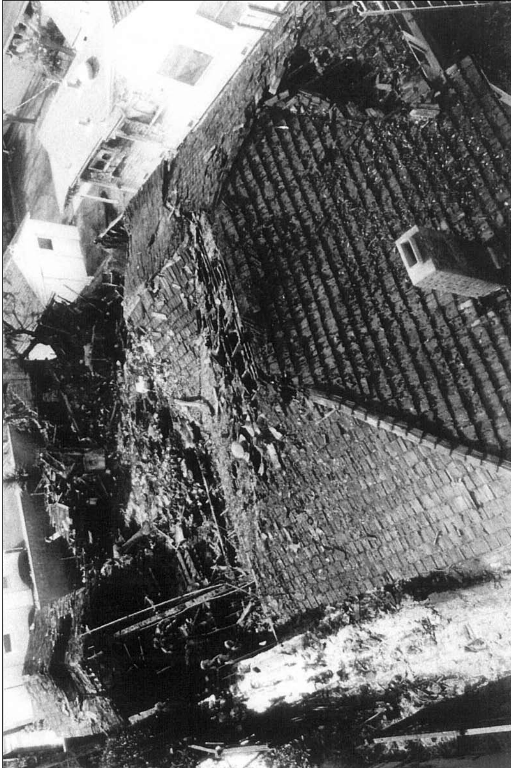
2. Looking south towards rear of house -- note area of second floor collapse
