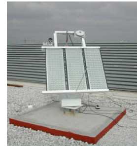
Figure 3. Three finished PV concentration modules installed in a two axis tracking system
