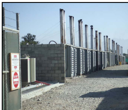
Figure 4.36. Expeditionary Power Plant.
