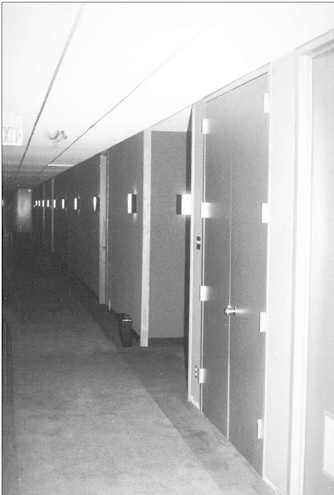
11. Fifth floor corridor looking toward rear of building. Electrical closet is in foreground. Elevator lobby and front stairway are around the corner to right.
