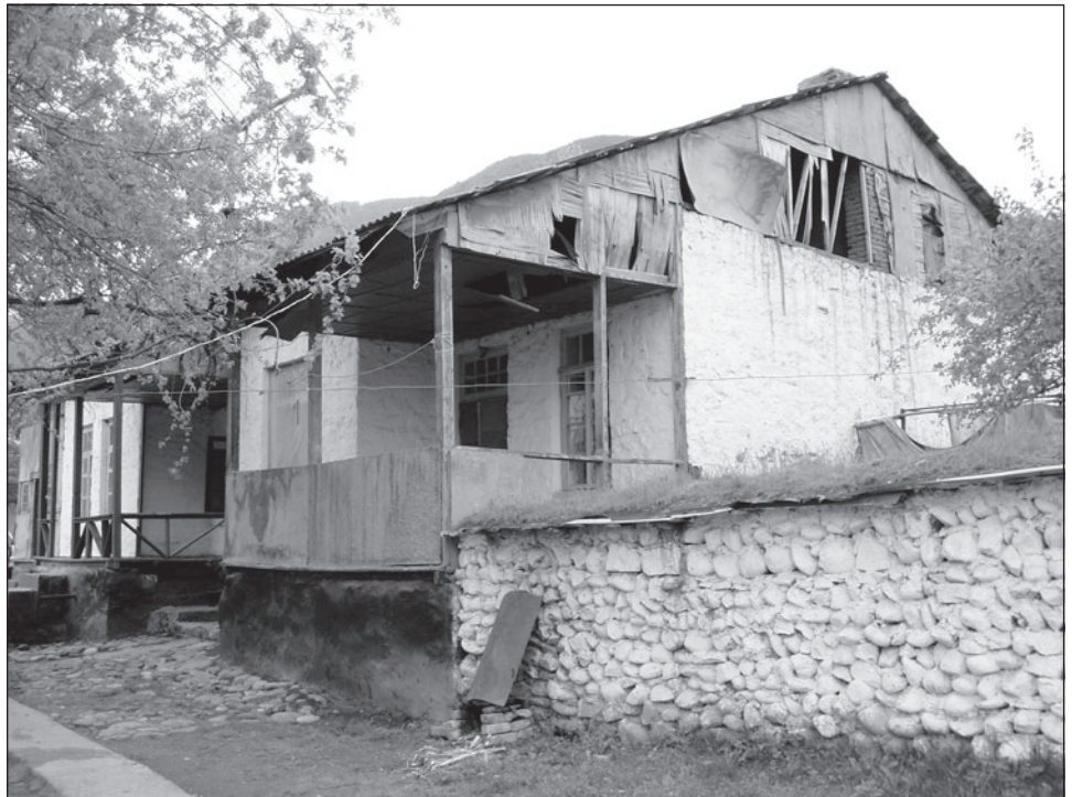
Figure 7: Khirmanjo, Tajikistan, Border Post Scheduled to Be Refurbished
