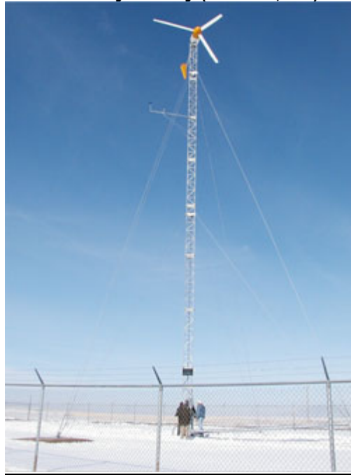
Photo 3: Turbine installed at Liberty County Maintenance Facility Source: NWSEED
