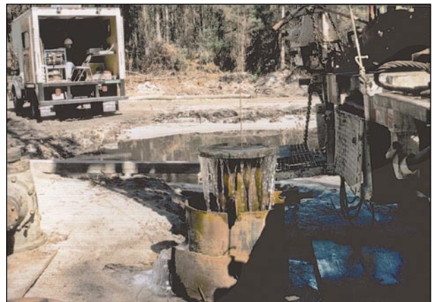
A public supply well in Glynn County is shown flowing at about 30 gallons per minute while spinner flowmeter logs were collected to estimate the percentages of water from different water-bearing zones. This well is completed in the confined surficial, upper Brunswick, and lower Brunswick aquifers, and the flowmeter logs help to quantify the ground-water contribution from each zone. Photo by Michael F. Peck, USGS.
