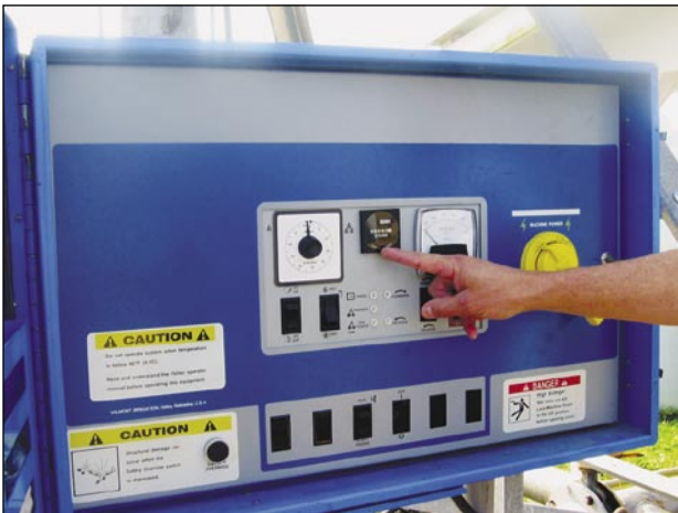
Control panel and time totalizer for monitoring usage of center-pivot irrigation system. Photo by L. Elliott Jones, USGS.
