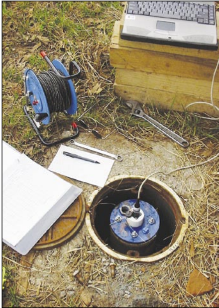
A downhole continuous recorder in Gwinnett County, Georgia, which is part of the ground-water-level monitoring network for an ongoing study. The equipment consists of a data logger, battery, and 15-pounds-per-square-inch transducer—all installed inside of a 6-inch-diameter casing. The recorder is set to collect data on an hourly basis, and processed and stored in National Water Information System. Photo by Alan M. Cressler, USGS.
