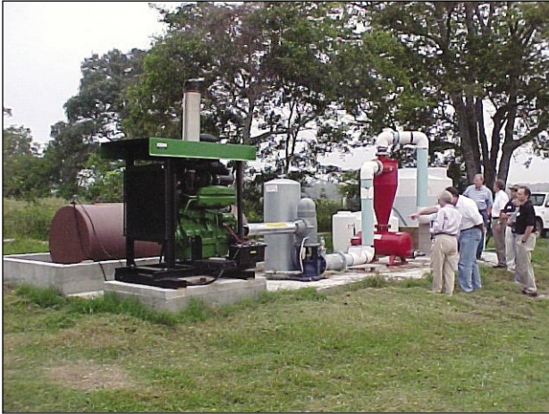
Chemigation/irrigation apparatus installed in well tapping the Upper Floridan aquifer southeast of Lake Seminole, Decatur County, Georgia. Well is 700 feet deep and was used in an aquifer-performance test. Photo by Lynn J. Torak, USGS.
