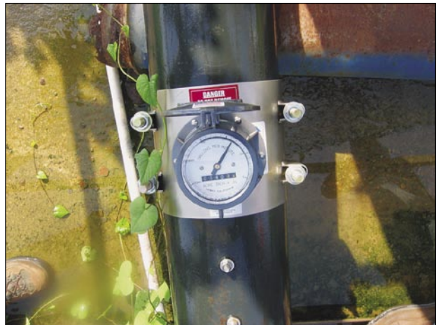
Flowmeter installed in discharge line of irrigation system. Photo by L. Elliott Jones, USGS.
