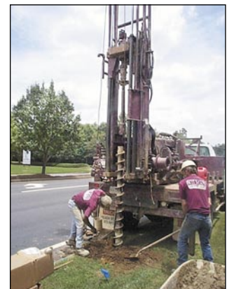
Drillers install a new regolith monitoring well. Photo by Phillip N. Albertson, USGS.
