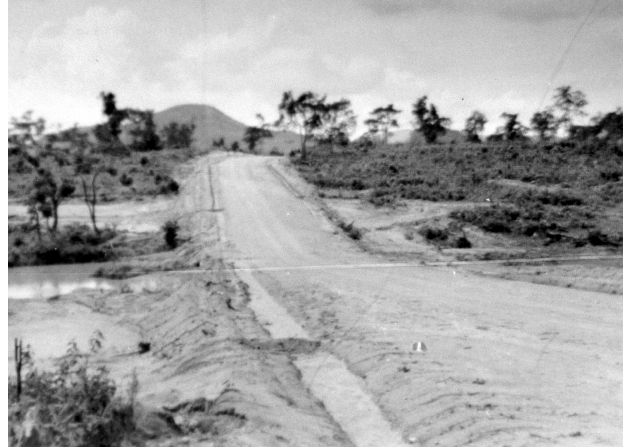
In May 1962 Company C of the 201st Engineer Battalion was constructing a road north from An Khe to Kannack.
