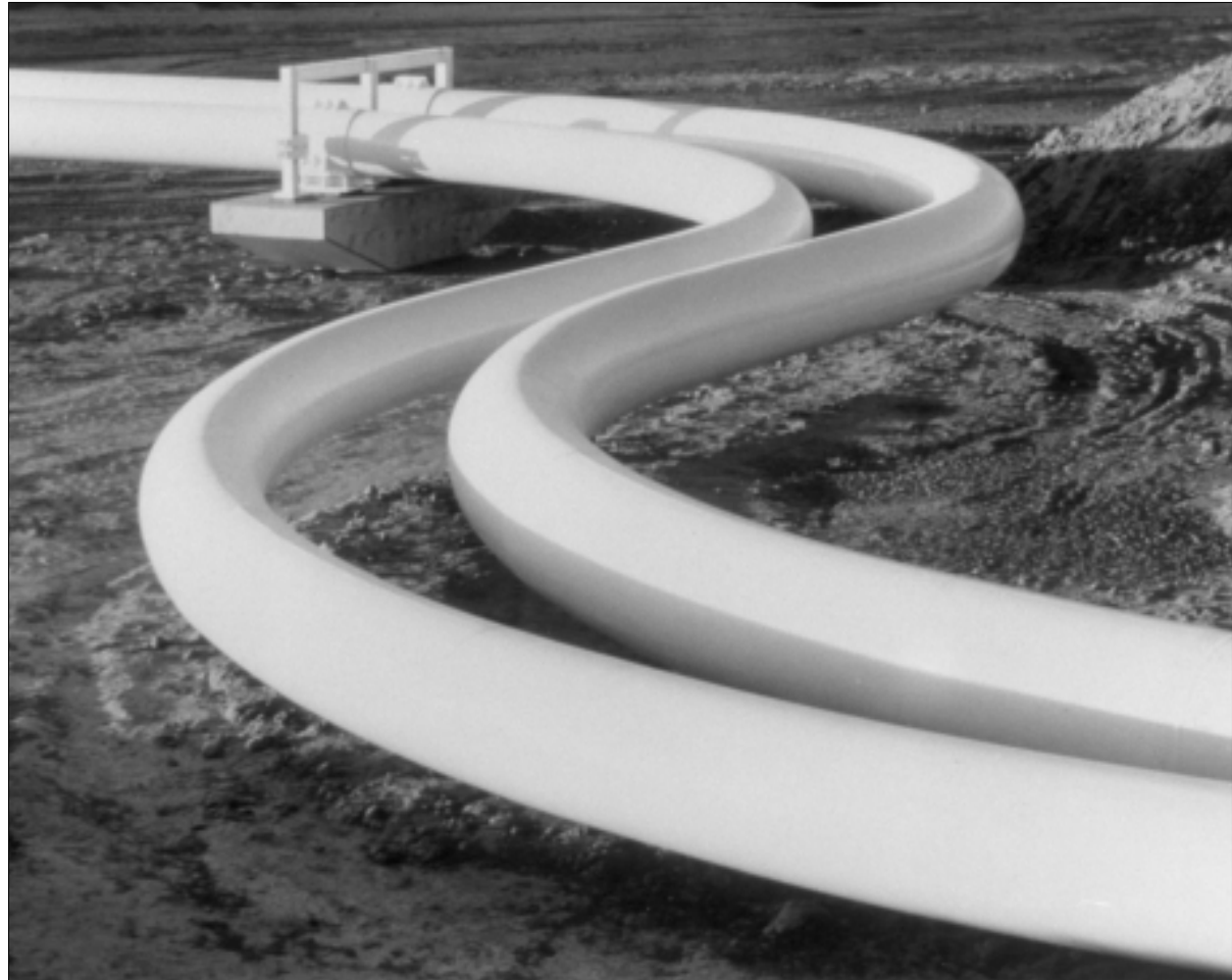
Natural gas pipeline, El Paso County, Texas. Source: U.S. Department of Energy.
