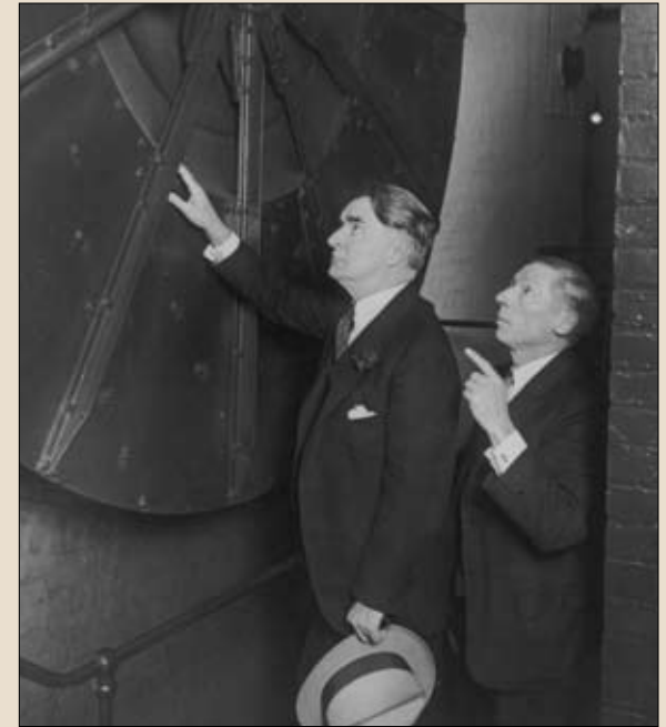
Senator Royal S. Copeland of New York (1923-1938), left, advocate for better air quality in the Senate, inspecting one of the ventilating fans that supply air to the Senate Chamber.
