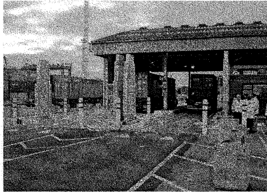
Figure 2. Radiation Portal Monitors in Felixstowe, U.K.
