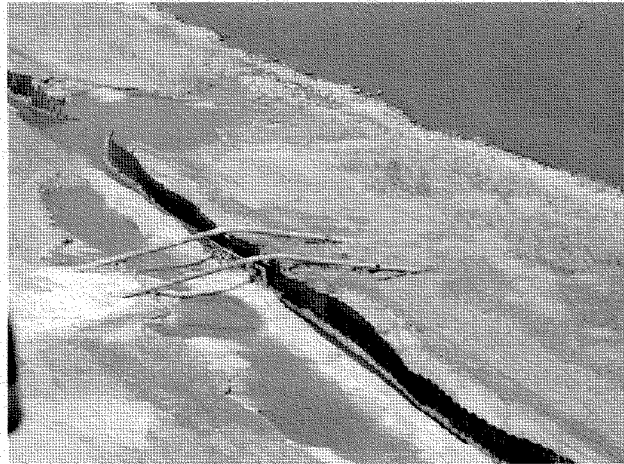
Figure 4.21: Levee failure on southwestern bank of MRGO between Bayou Bienvenue (where barge is aground on I-wall) and Bayou Dupree. Note severe erosion and scouring (L. Harder, October 14, 2005).
