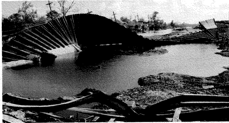
Figure 4.10: Overturned I-wall system at north breach of Lower Ninth Ward (J. Wartman, October 4, 2005).
