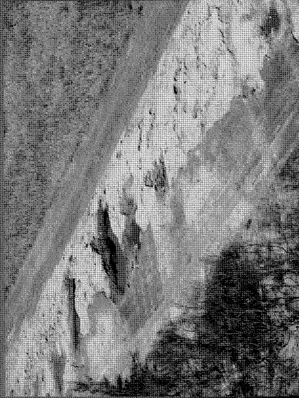
Overtopped Embankment (Sand Core)
