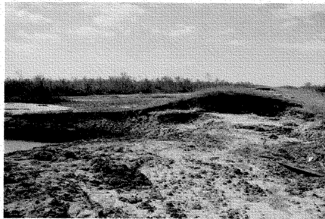
Figure 4.24: Failure of earth levee on southwest bank of MRGO adjacent to the Bayou Dupree gate (L. Wooten, October 6, 2005).
