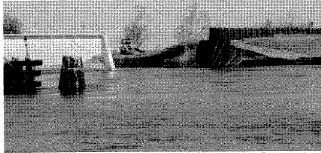
Figure 4.13: Sheet pile breach at the Bayou Bienvenue Gate (J. Wartman, October 5, 2005).
