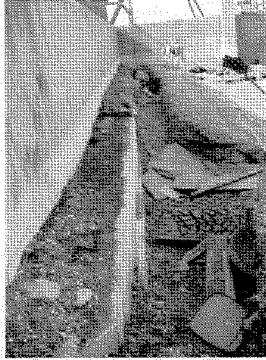
Figure 4.8: A scoured, but nevertheless well-performing "T-wall" levee section located near the north breach of the Lower Ninth Ward (J. Wartman, October 4, 2005).
