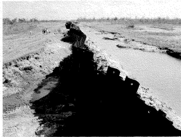
Figure 4.20: Failure of earth levee with steel sheetpile barrier on the southeast bank of the MRGO. Note severe erosion and scour (L. Wooten, October 6, 2005).
