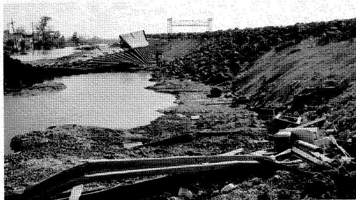
Figure 4.11: Looking south along the north breach repair at the Lower Ninth Ward (J. Wartman, October 4, 2005).
