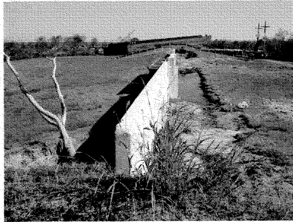
Figure 4.15: Scour near Bayou Bienvenue Gate site (L. Wooten, October 5, 2005).
