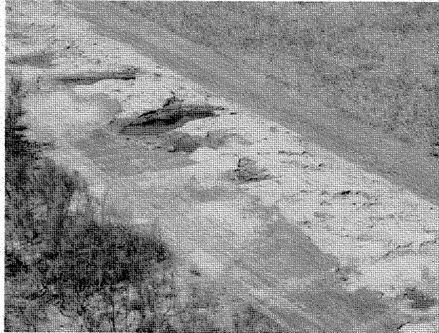
Figure 4.25: Overtopping obliterated earth levee along southwestern bank of MRGO, within two miles southeast of Bayou Dupree. Note deep scour at the levee foundation level (L. Harder, October 14, 2005).
