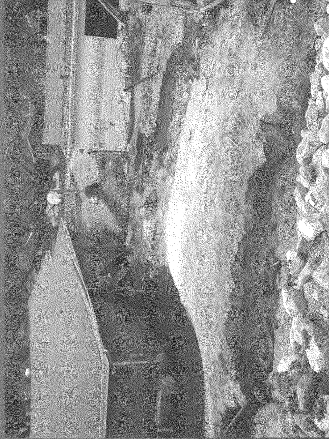
London Avenue Canal, North Breach
