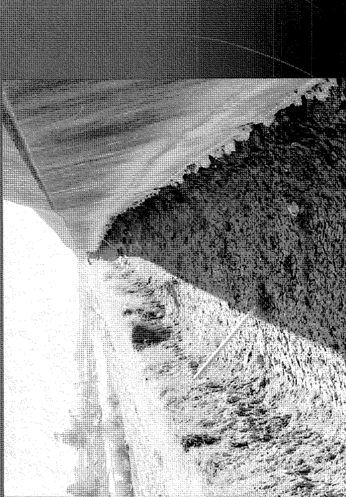
Inner Harbor Navigation Channel Back Scour at Lower 9th Ward
