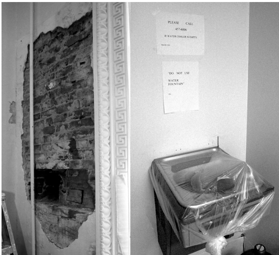
Figure 6: Water Damage in EEOB in Washington, D.C., and Covered Water Fountain with Posted Warning Against Drinking the Water in FOB 3, Suitland, Md.
