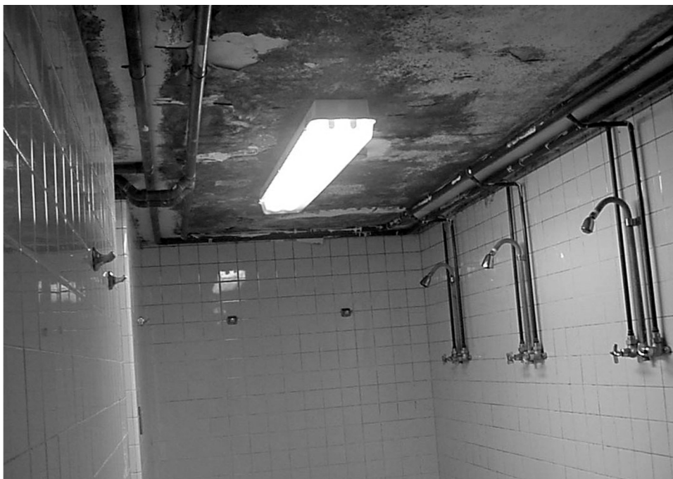
Figure 5: Shower Ceiling Damage at Fort Jackson, S.C., Recruit Barracks
