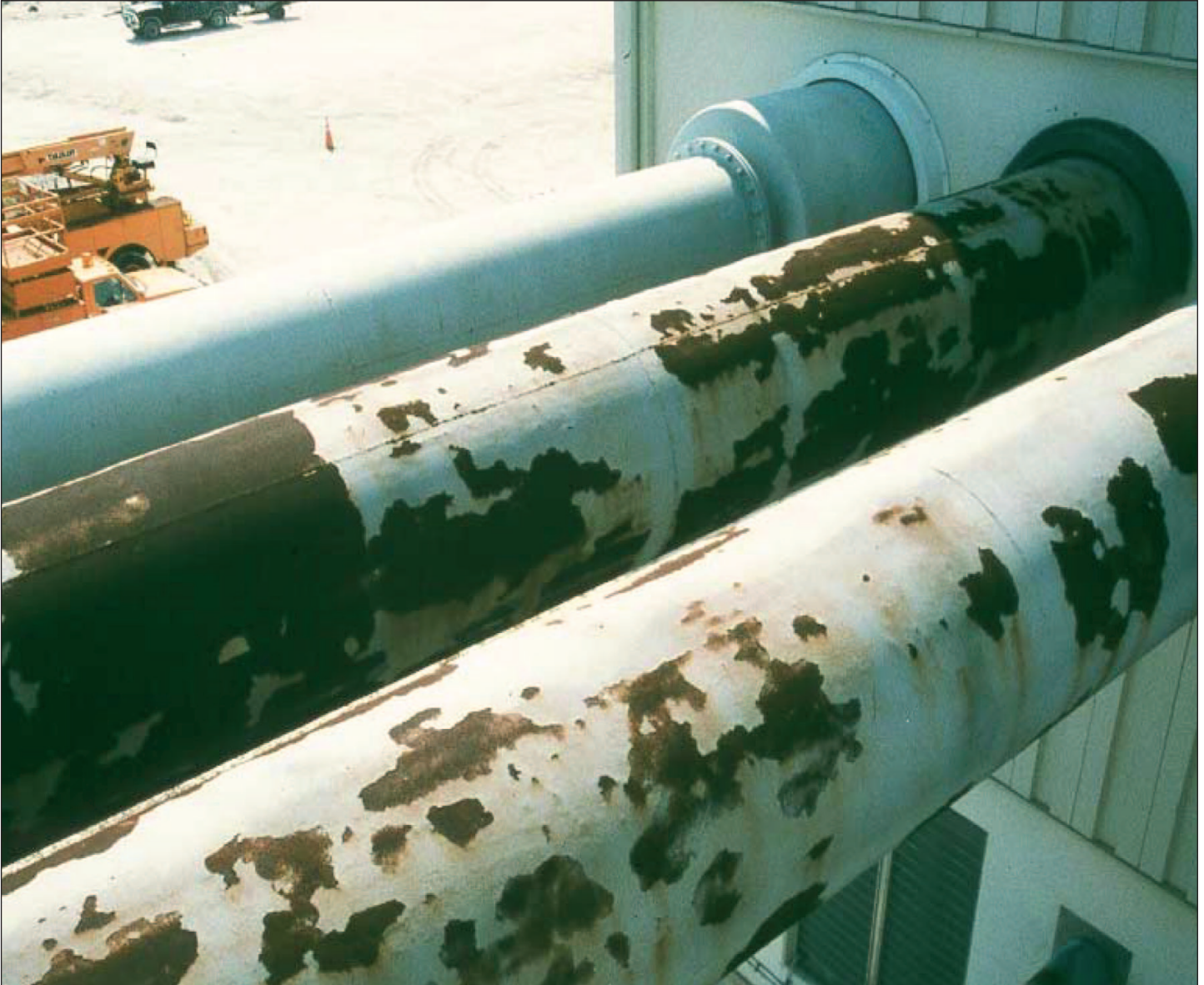
Figure 11: Corrosion on High Temperature Pipelines at Air Force Tracking Facility Antigua, West Indies
