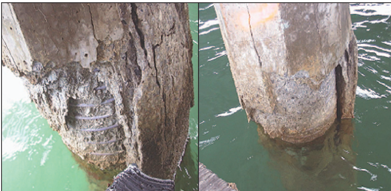
Figure 2: Corroding Bridge Columns at Naval Station Pearl Harbor, Hawaii
