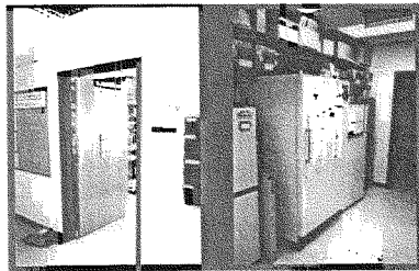
Figure 1. Open and Accessible Biological Agent Storage Room
