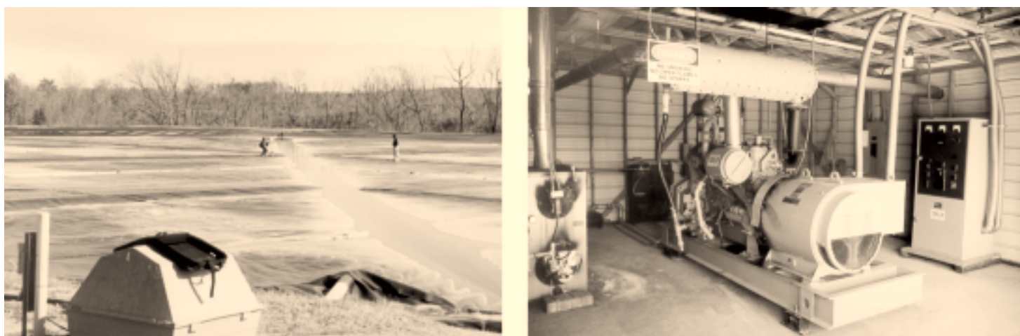
Figure 7: Covered Lagoon to Capture Methane Gas and Electric Generator and Water Heater Powered by This Methane
