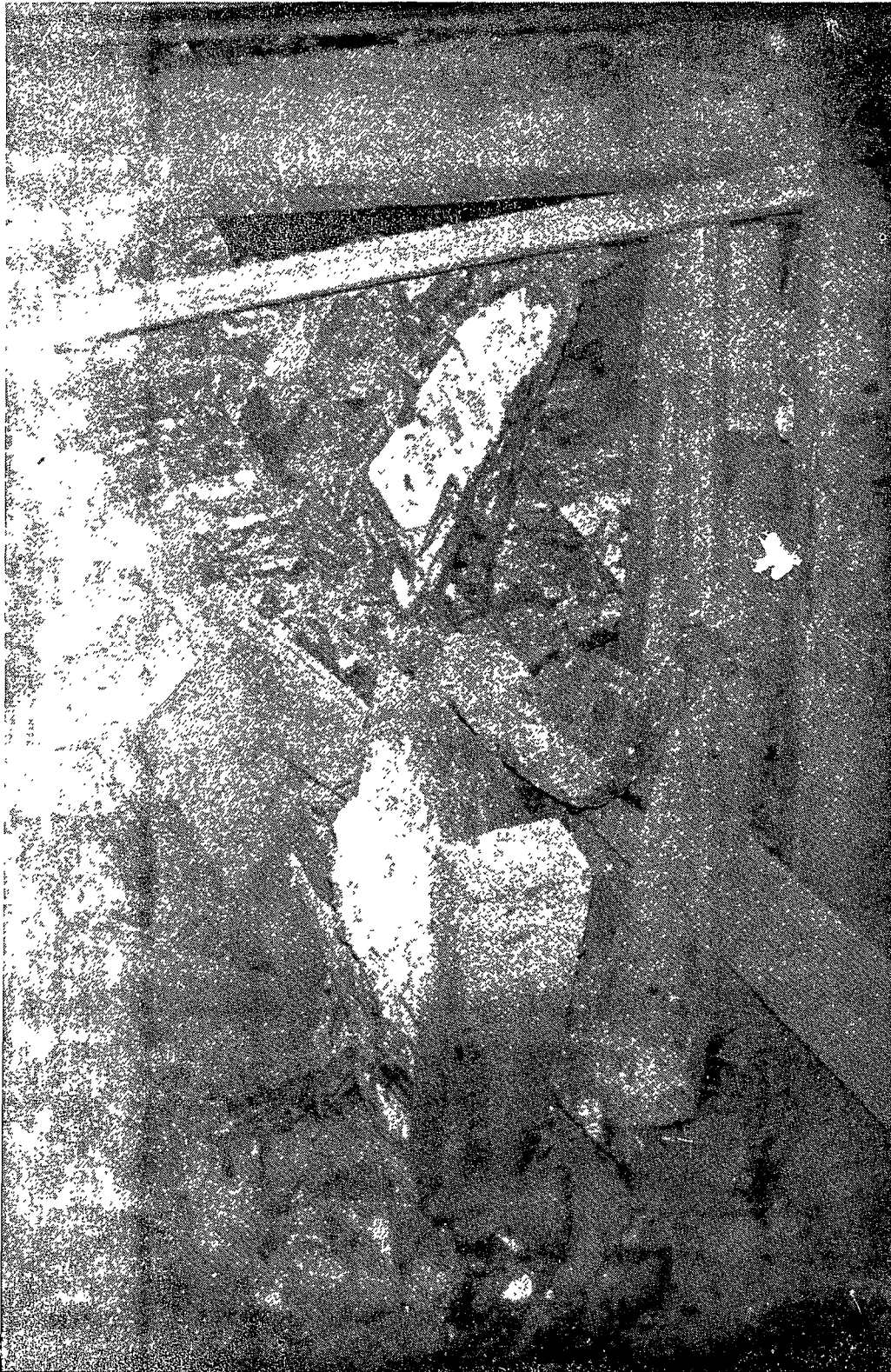
Fall of roof in a timber-supported working area of an underground mine. Employees were not in the area when the accident occurred.
